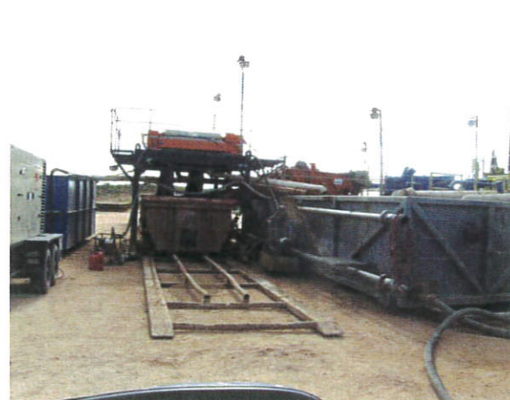
Above: Centrifugal Closed Loop System
