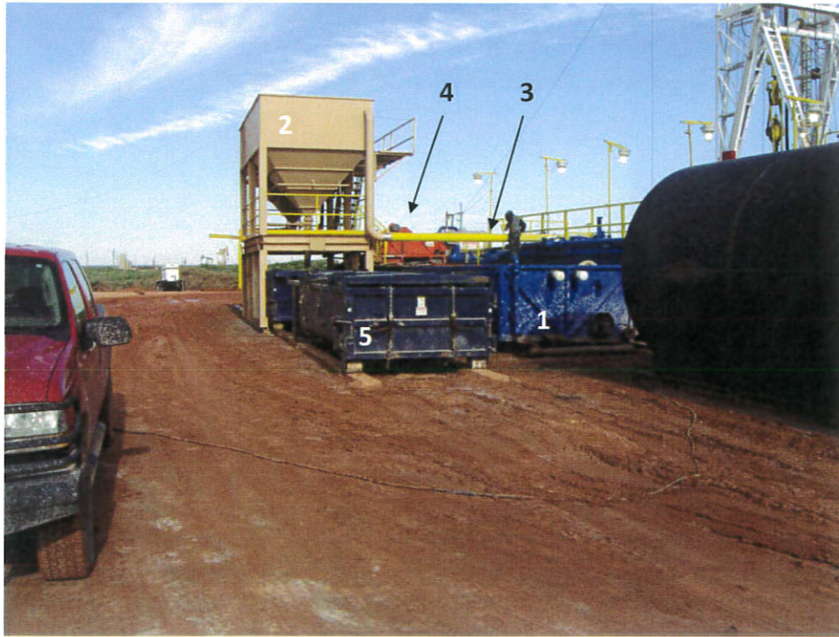
Closed Loop Drilling System: Mud tanks to right (1) Hopper in air to settle out solids (2) Water return pipe (3) Shaker between hopper and mud tanks (4) Roll offs on skids (5)
