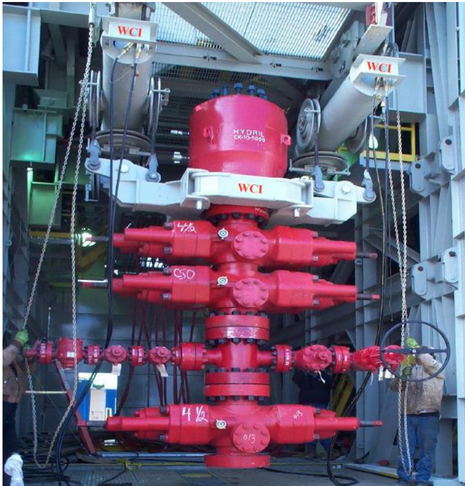
Figure 3. BOP handling system
