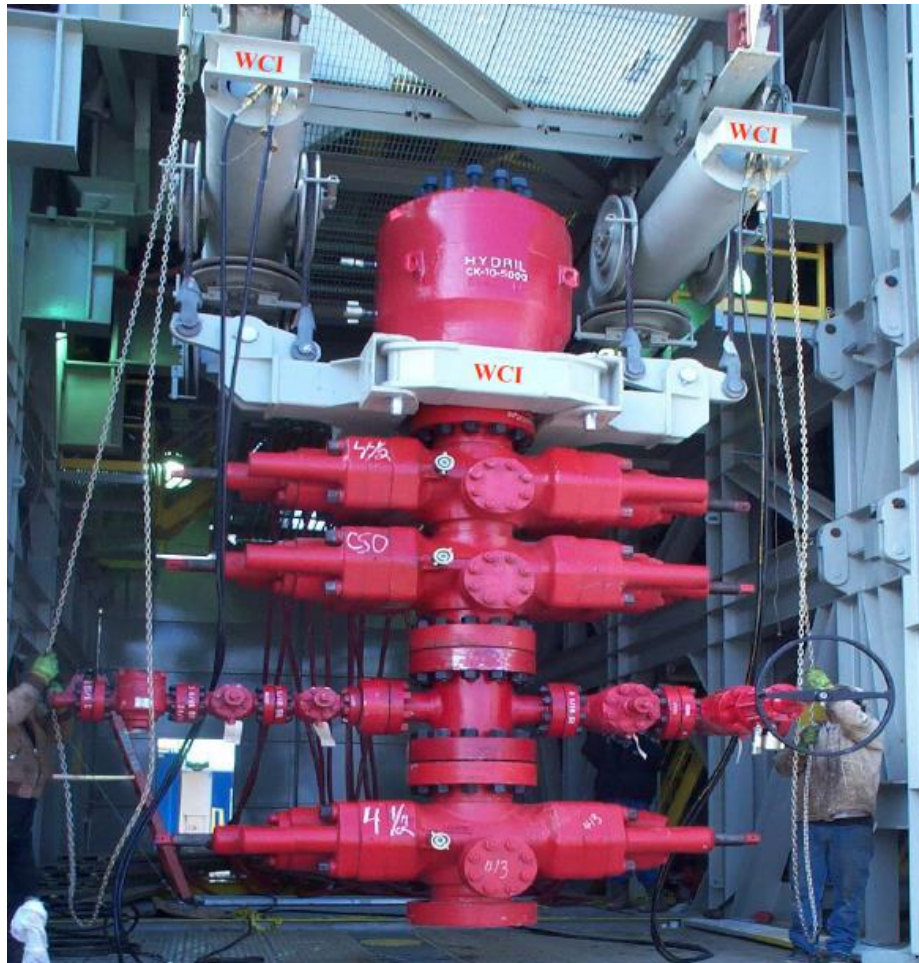
Figure 3. BOP handling system
