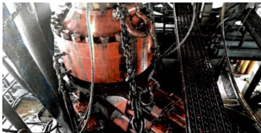
Figure 1: Winch System attached to BOP Stack
