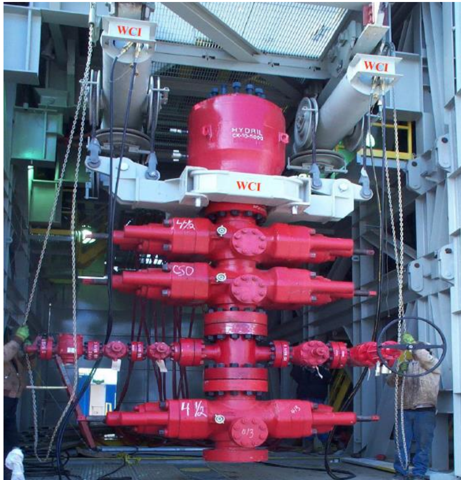
Figure 3. BOP handling system
