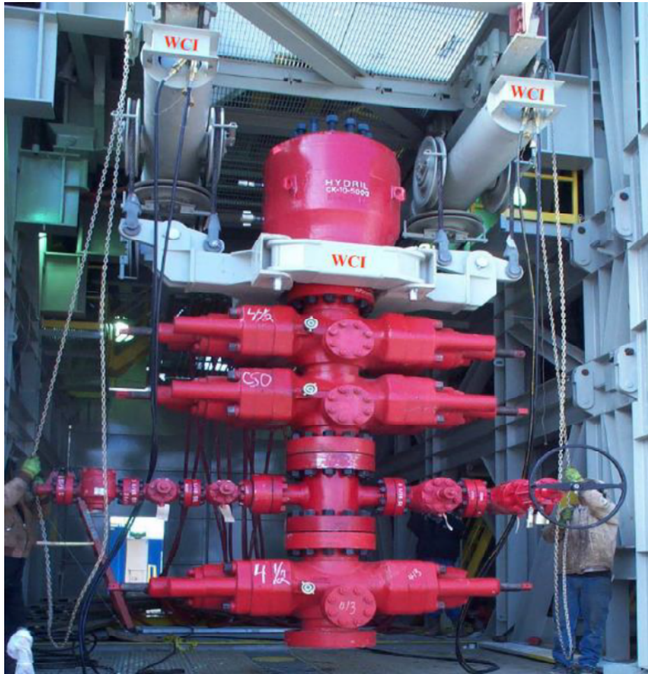
Figure 3. BOP handling system
