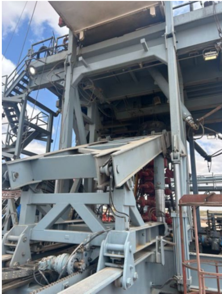
Figure 3: BOP handling system
