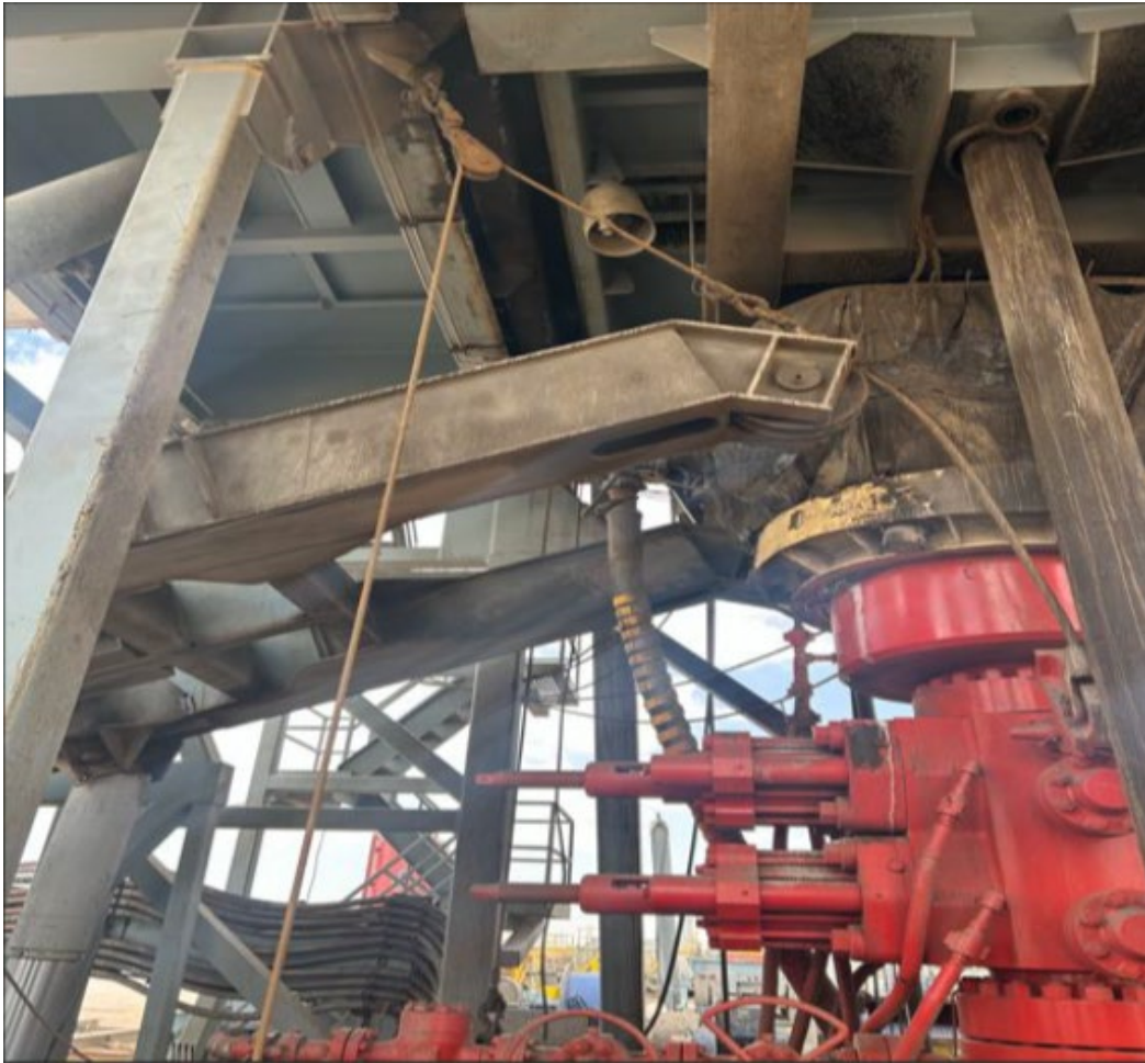
Figure 4: BOP handling system
