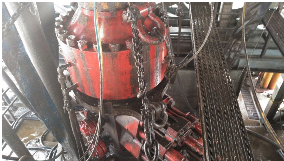
Figure 1: Winch System attached to BOP Stack
