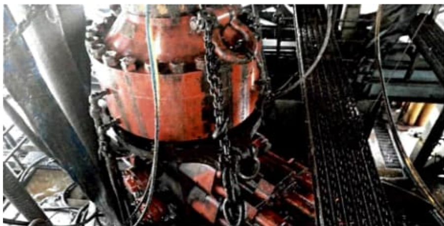
Figure 1: Winch System attached to BOP Stack
