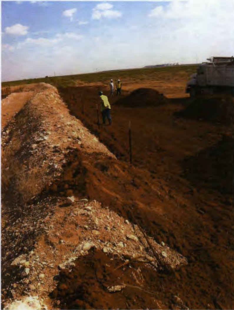
The entire excavated area is back filled with clean material and additional material is placed to enhance the top soil of the scraped area.
