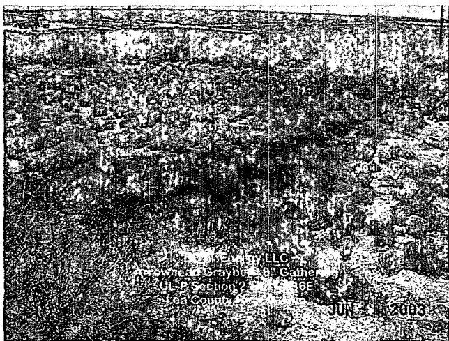
Leak origin, looking east-southeast.
