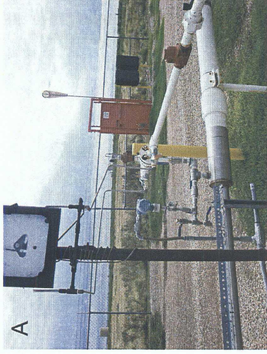
A. Pipeline at Dagger Draw Plant
