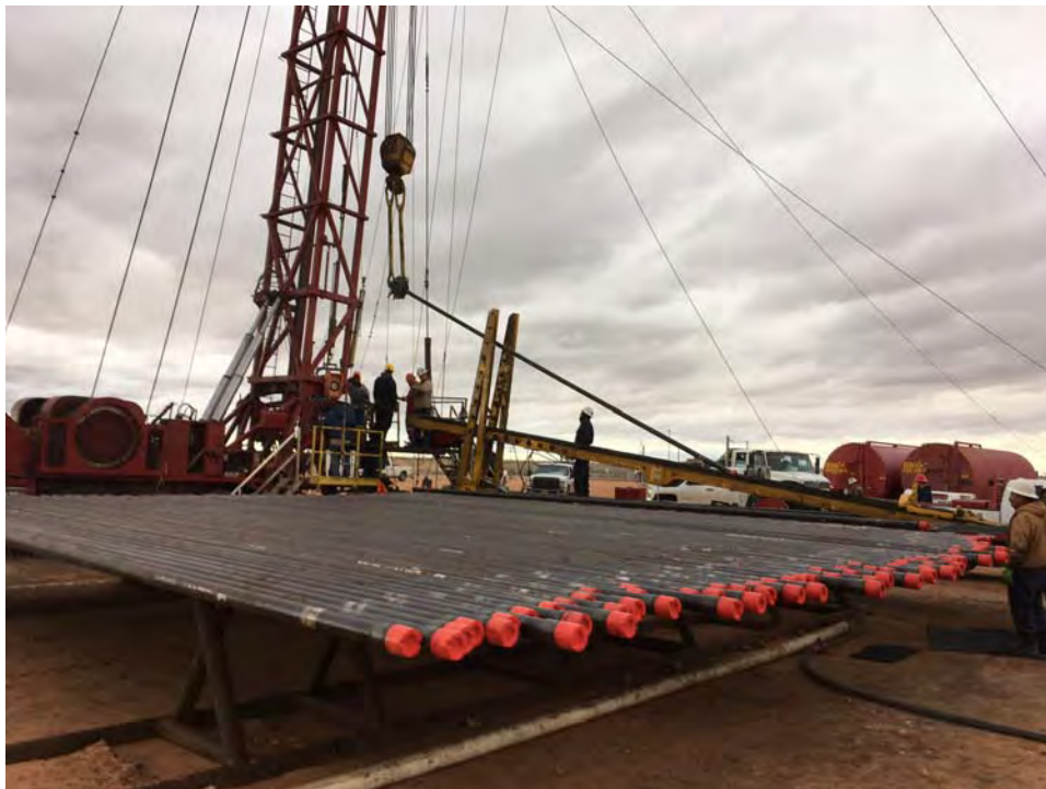
Figure 1: Eighty-four strings of tubing left on the rack to be placed in the hole.
