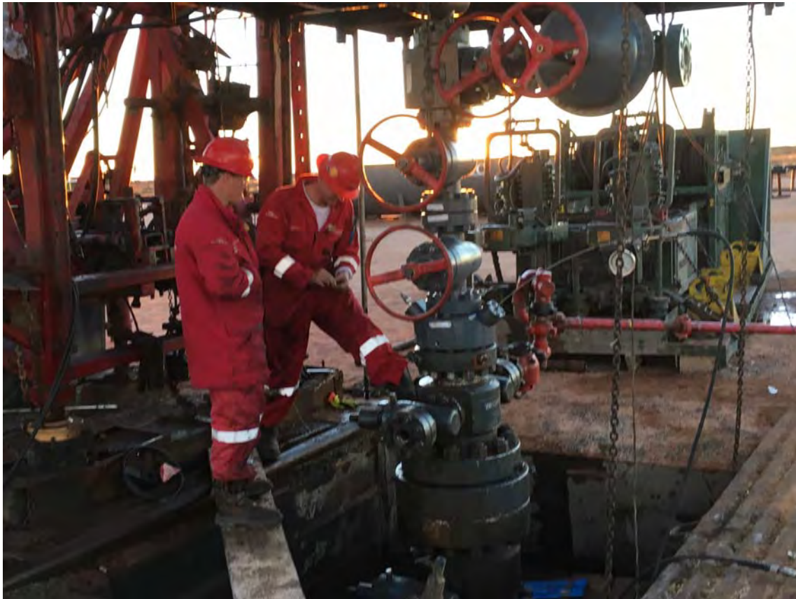
Figure 1: Christmas tree installed. Halliburton is making final adjustment to P/T gauge data line.
