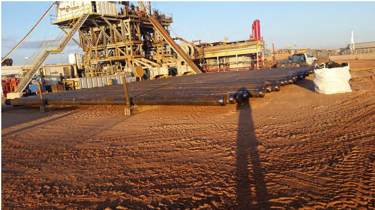
Figure 1: Battle Testing unit Completing CIT and 13 3/8-inch surface casing on the rack
