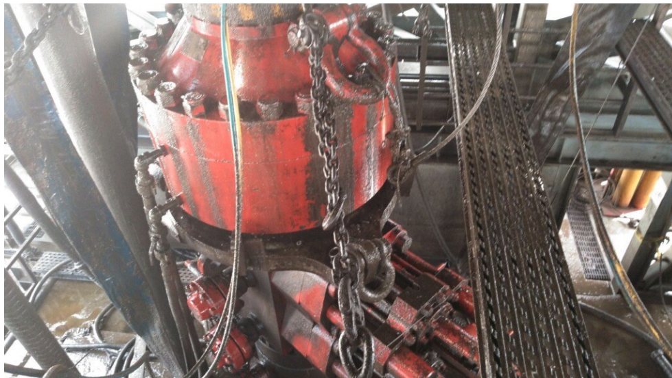
Figure 1: Winch System attached to BOP Stack
