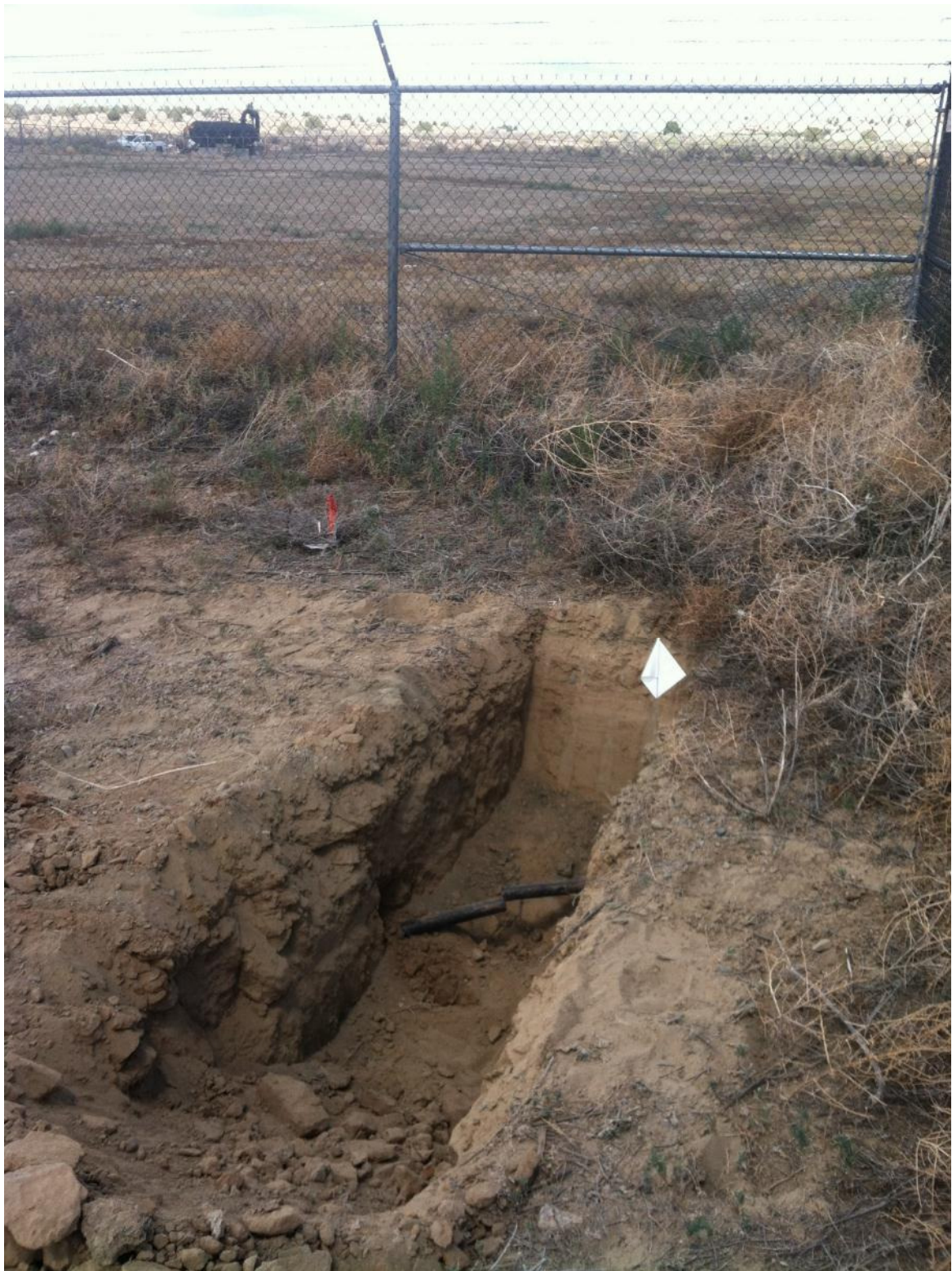
Electrical supply disconnect.
