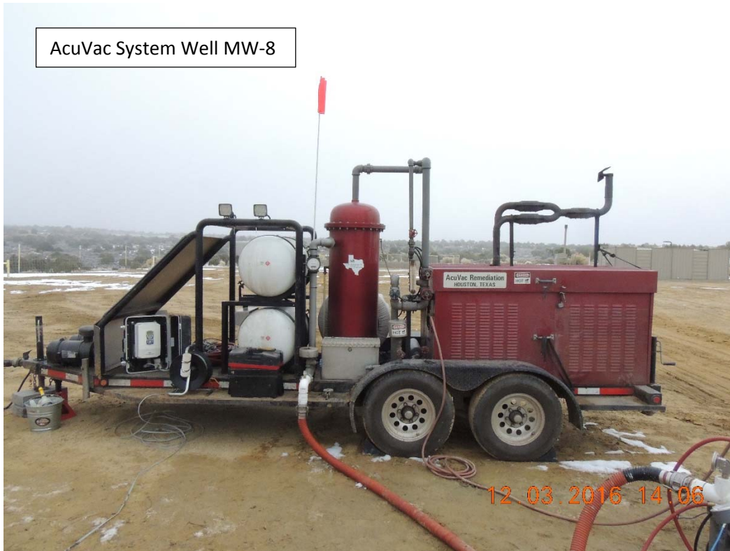
AcuVac System Well MW-8
