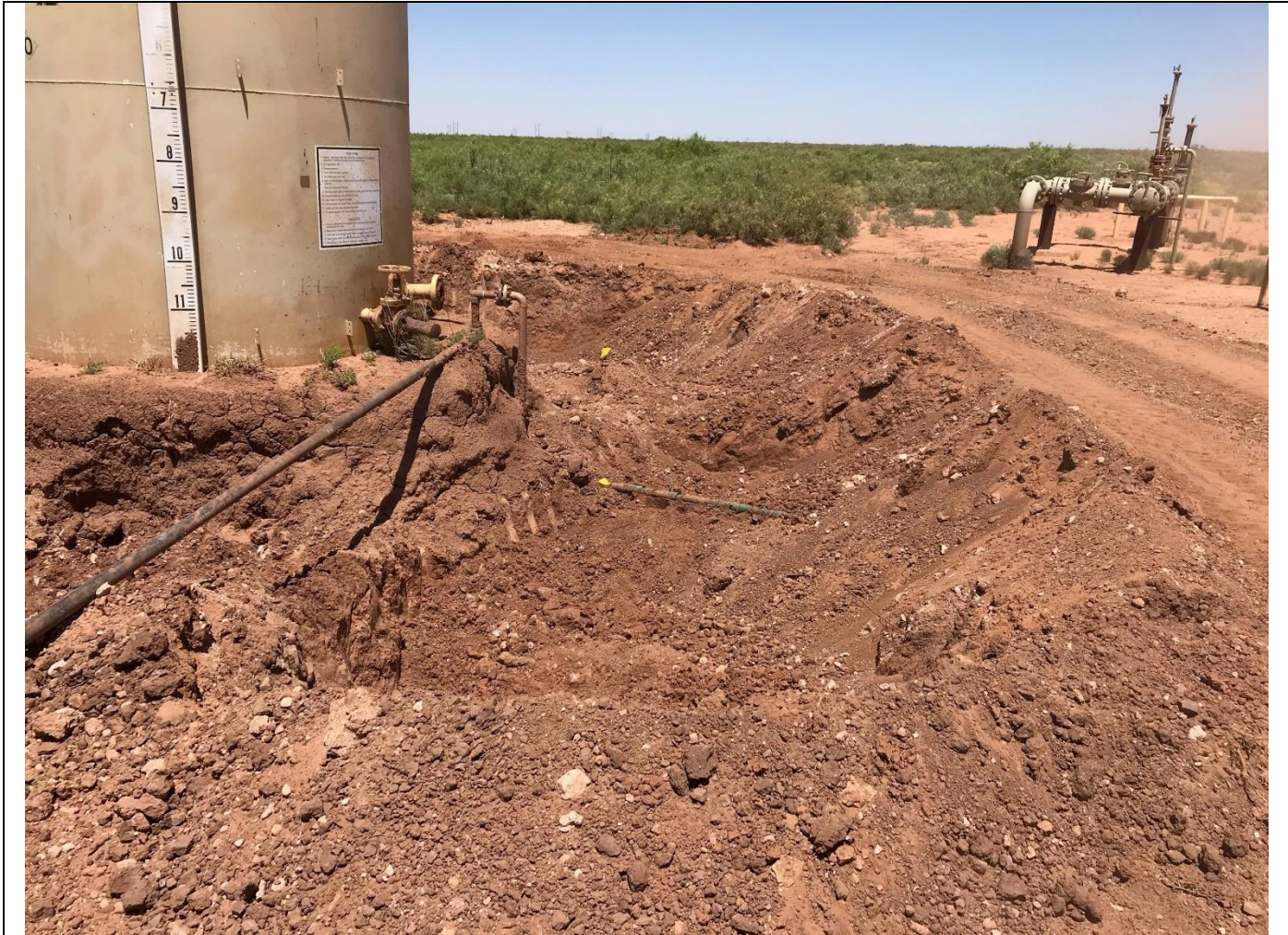
Eastern view of the excavation extent on the south side of the tank battery during excavation activities.
