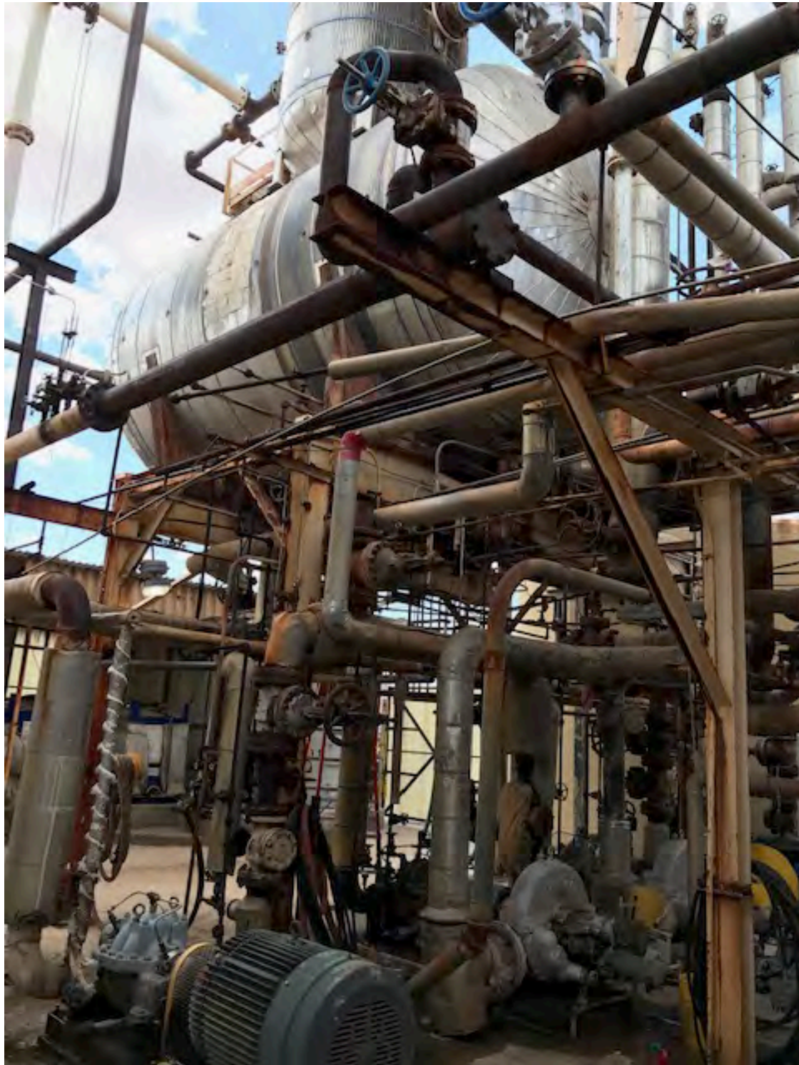
Step 3: Boiler water de-aeration unit.
