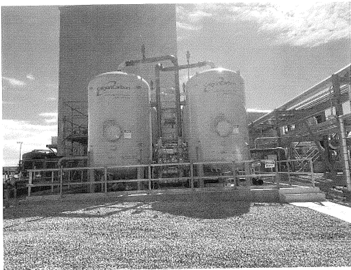
Photo 3: Updated carbon treatment system piping manifold.
