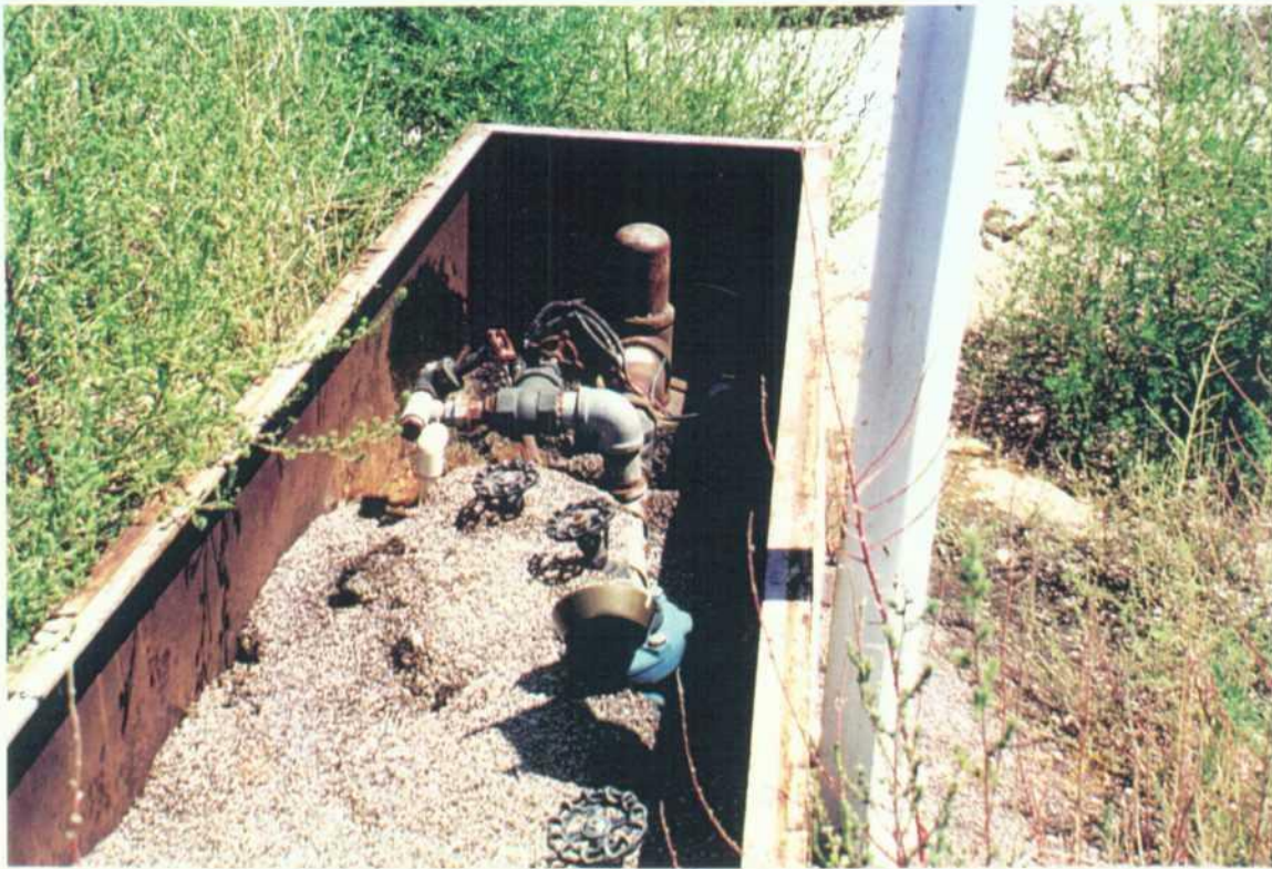
3. Plant Water Well
