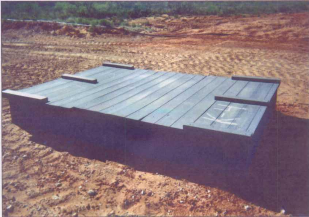
New K-4 Junction Box Located 50 ft West of Old Box Locations
