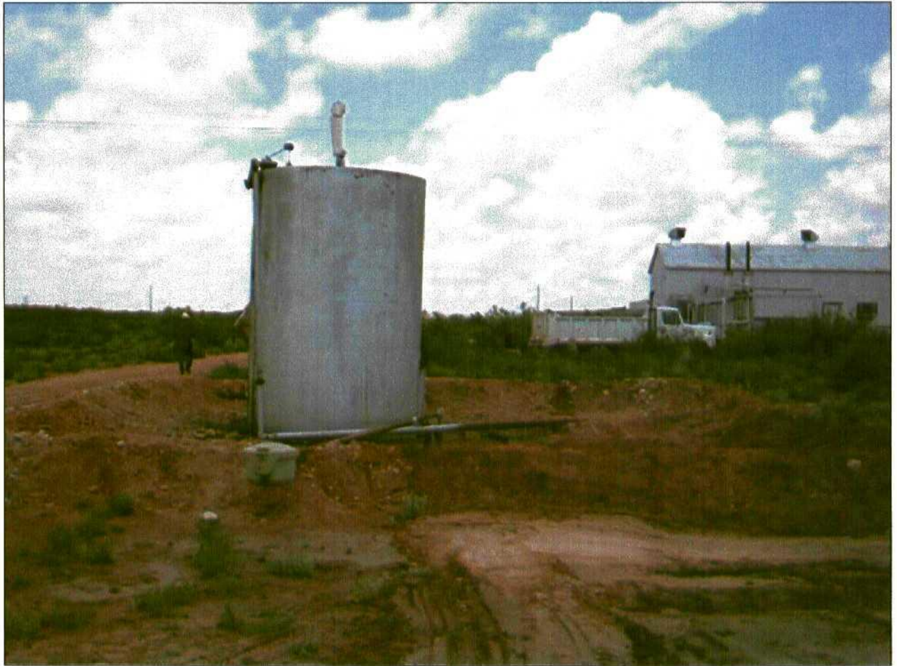
FIGURE 2. Lusk Compressor Station Slop Oil Tank (40' x 40')
