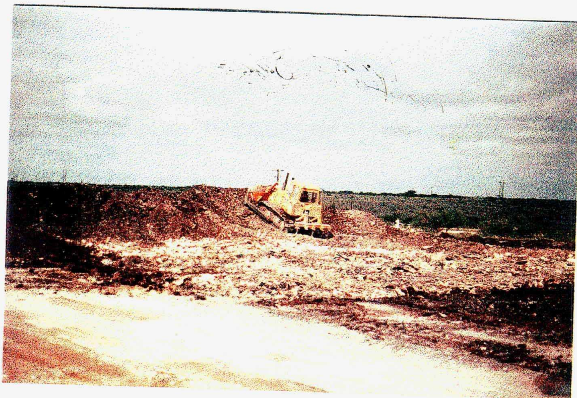
14/ AMERADA HESS NMGSAU BATTERY #1 FIRST STAGE OF PROJECT
