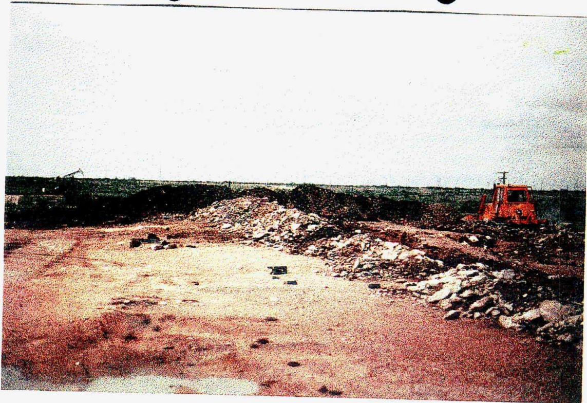
14/ AMERADA HESS NMGSAU BATTERY #1 FIRST STAGE OF PROJECT
