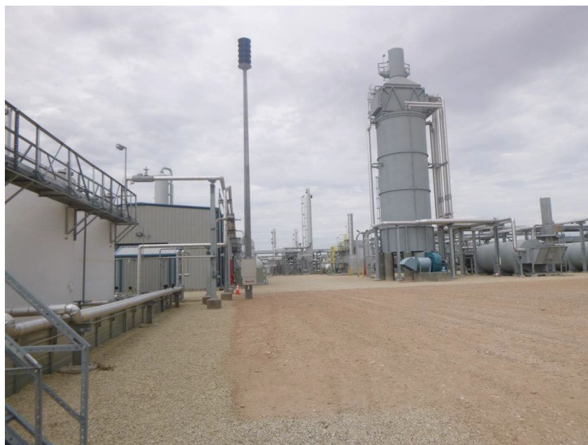
General equipment and piping on the central portion of the facility, facing north.
