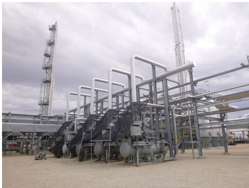
General equipment and piping on the southern portion of facility, facing east.
