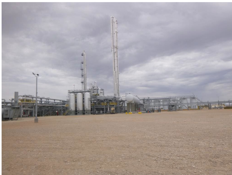
General equipment and piping on the northern portion of the facility, facing north.
