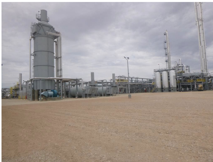
General equipment and piping on the central portion of the facility, facing northwest.
