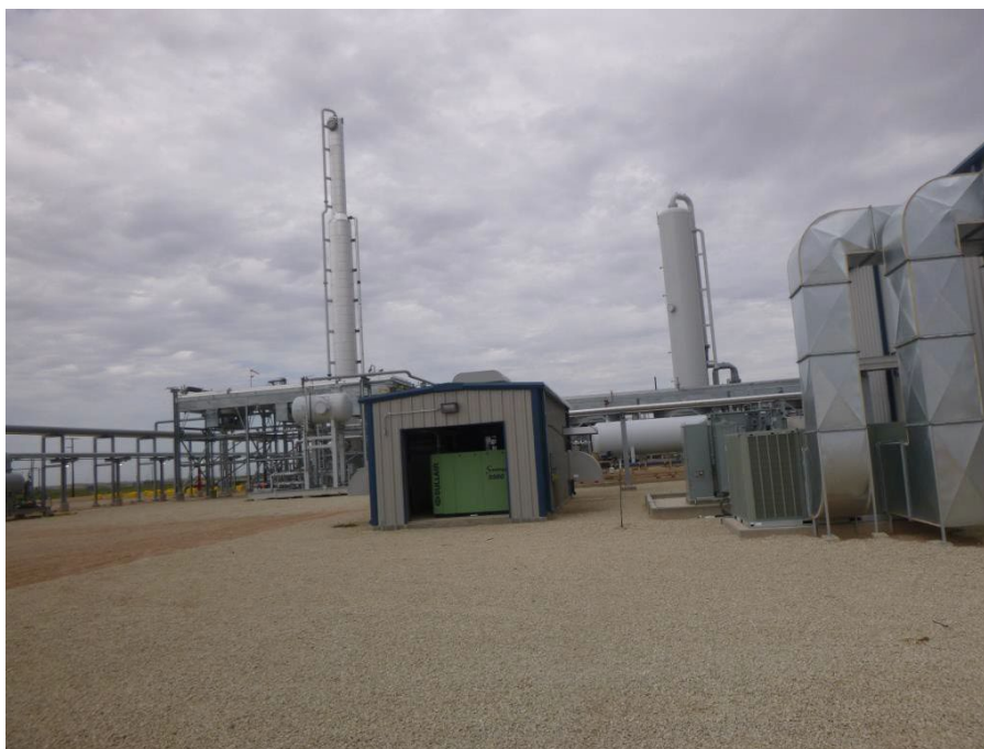
View of general equipment and piping on southern portion of the facility, facing west.
