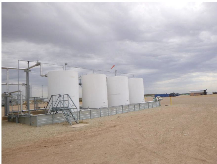
View of Main Containment 4 with metal dike containment, facing southeast.
