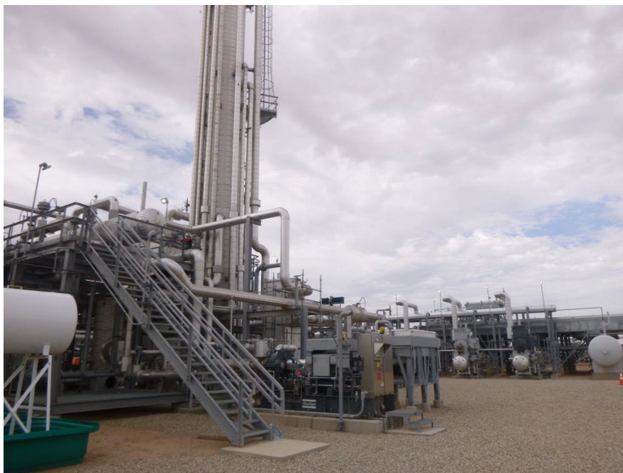
General equipment and piping on the central portion of the facility, facing southeast.
