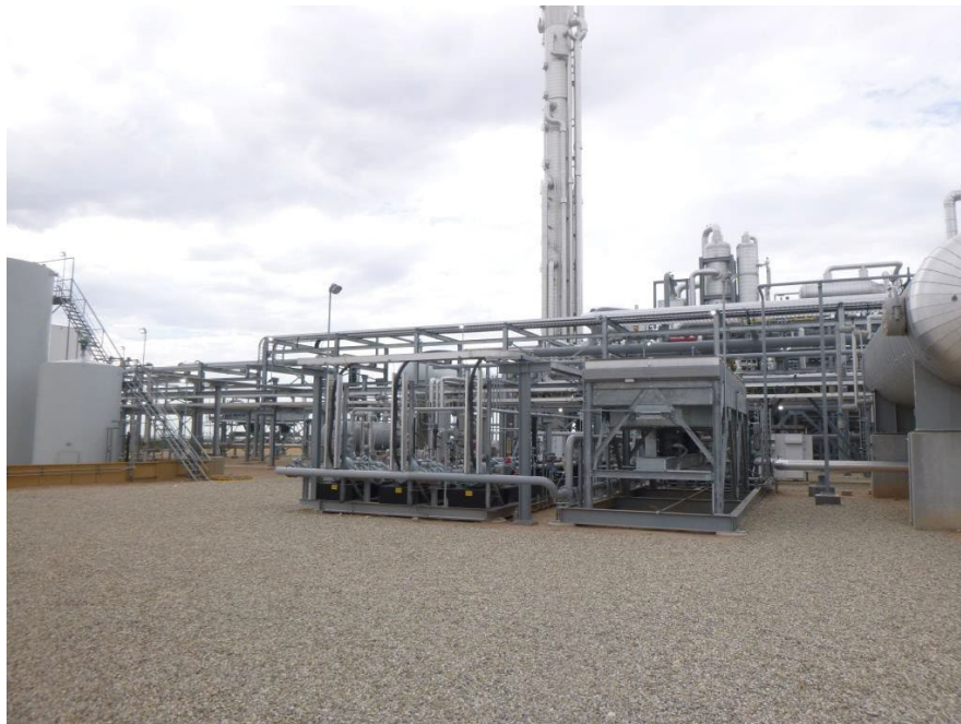
View of facility piping associated with Main Containment 1, facing north.
