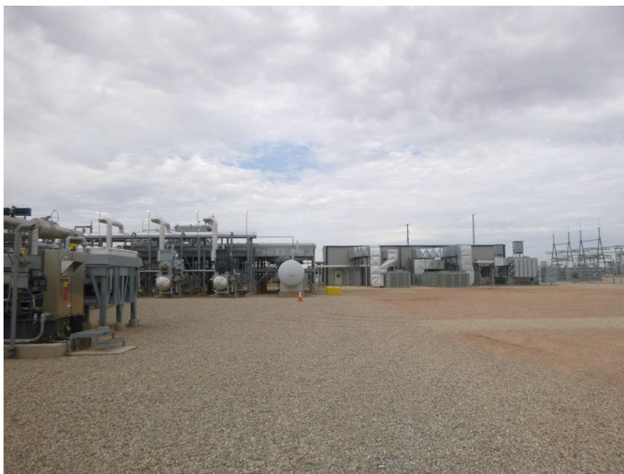
General equipment and piping on the northwest portion of the facility, facing west.
