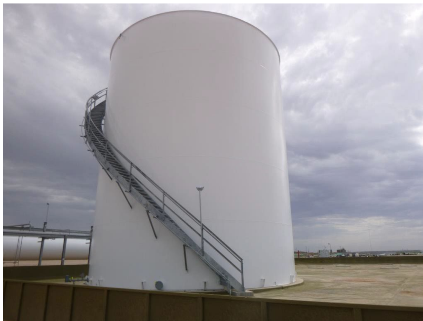
View of Main Containment 2 with metal dike containment, facing southeast.
