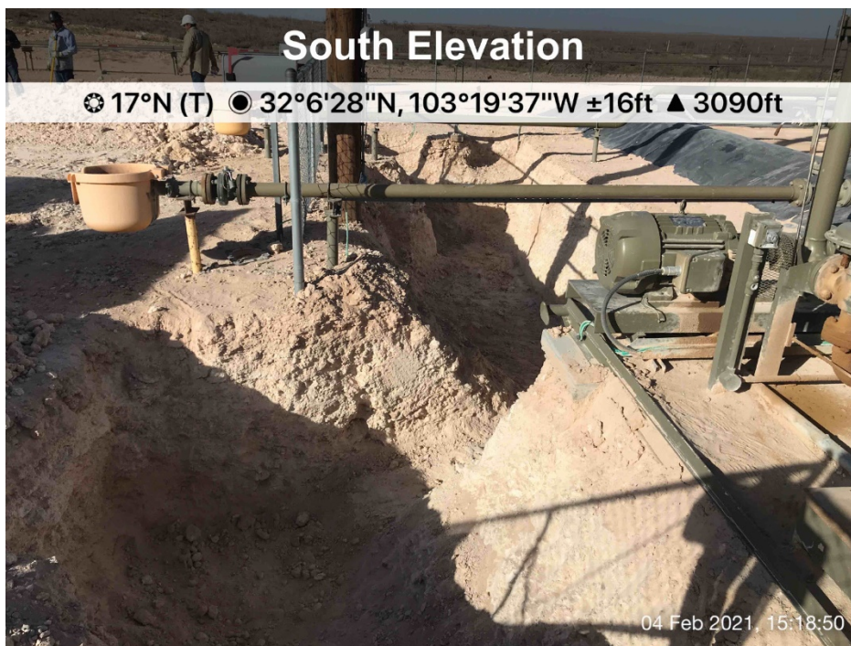
Soil excavated to a depth of 4.1 feet bgs encompassing C-5 and C-6, February 4, 2021
