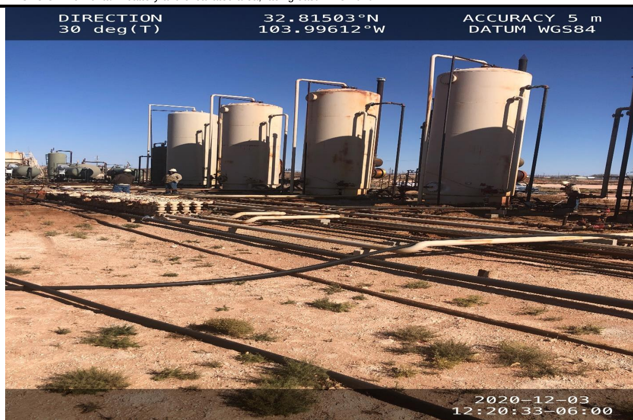
PHOTO 4: View of tank battery and pipes, facing north. 12-3-2020
