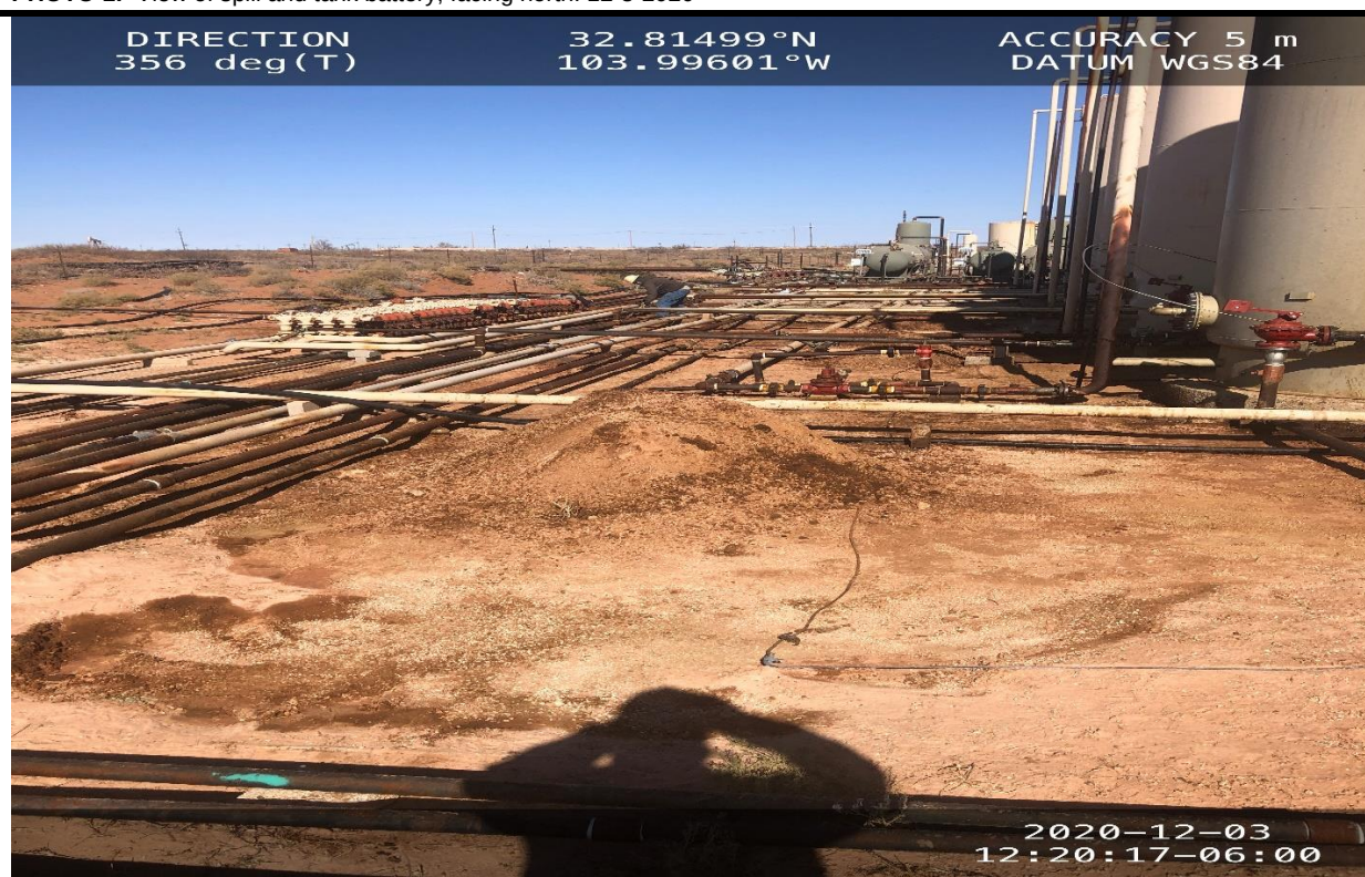
PHOTO 2: View of spill and tank battery, facing north. 12-3-2020
