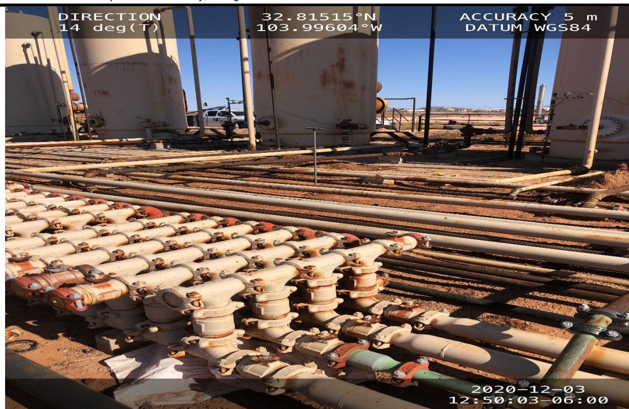
PHOTO 6: View of tank battery and connectors, facing north. 12-3-2020
