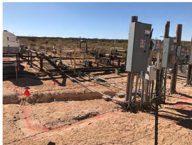
Photograph 8: South facing view of equipment in release area.
