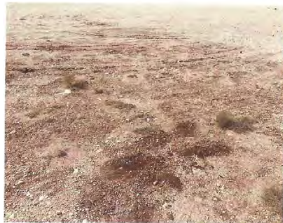
Large release was noted under gravel next to power disconnect. Contamination was seeping up through top layer.
