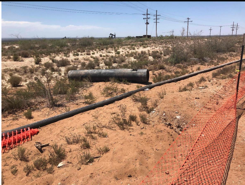
PHOTO 4: View of pipe that was struck and removed, facing Northwest. 7/6/2020
