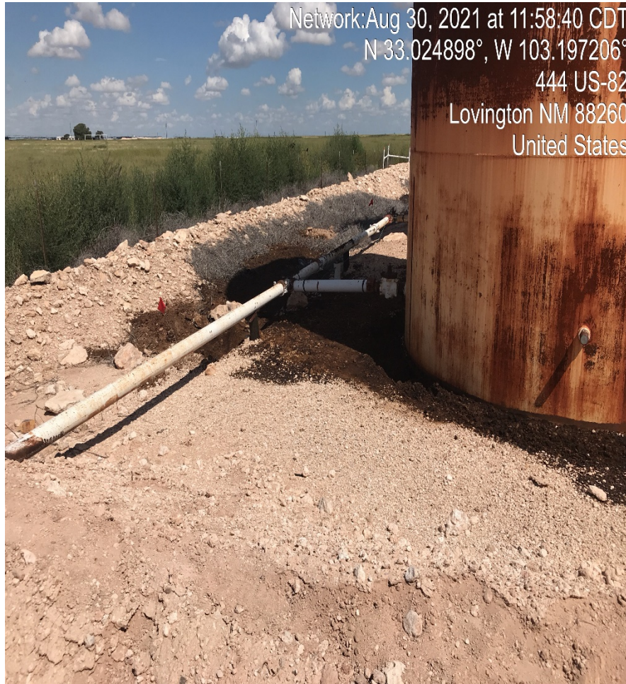
View North – Origin of spill. Cause of the release is due to corrosion on associated piping. Note a portion of the spill flow path (dark brown staining) within the release footprint.
