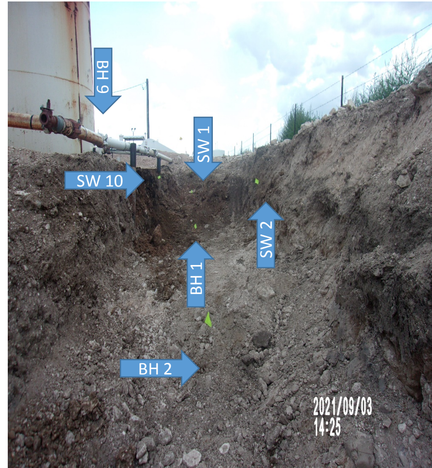
View South – Sample locations Bottom Hole 1 (3' EB), Bottom Hole 2 (4' EB), Bottom Hole 9 (1' EB), Side Wall 1, Side Wall 2 and Side Wall 10 (flagged). Blue arrows identify pin flags.
