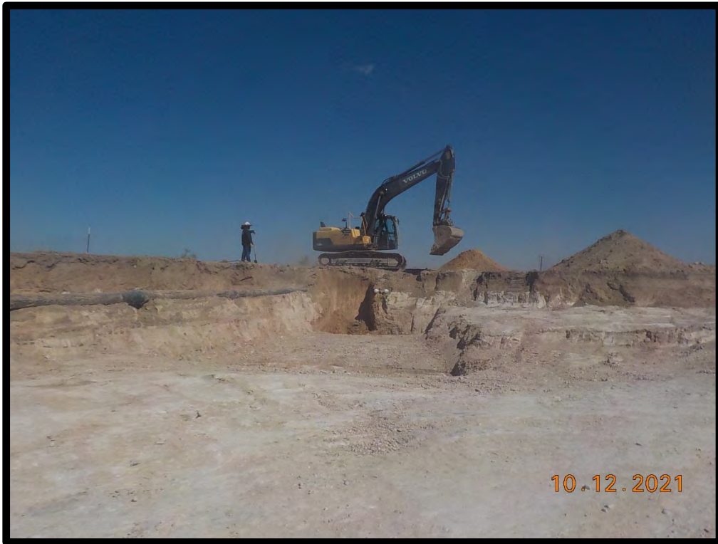
PHOTOGRAPH NO. 8 – A view of the on-going soil removal operations along the northern wall of the Western Impact/Excavation Area in the vicinity of the two PVC lines. (Approximate GPS coordinates 32.682723, -104.500133)
