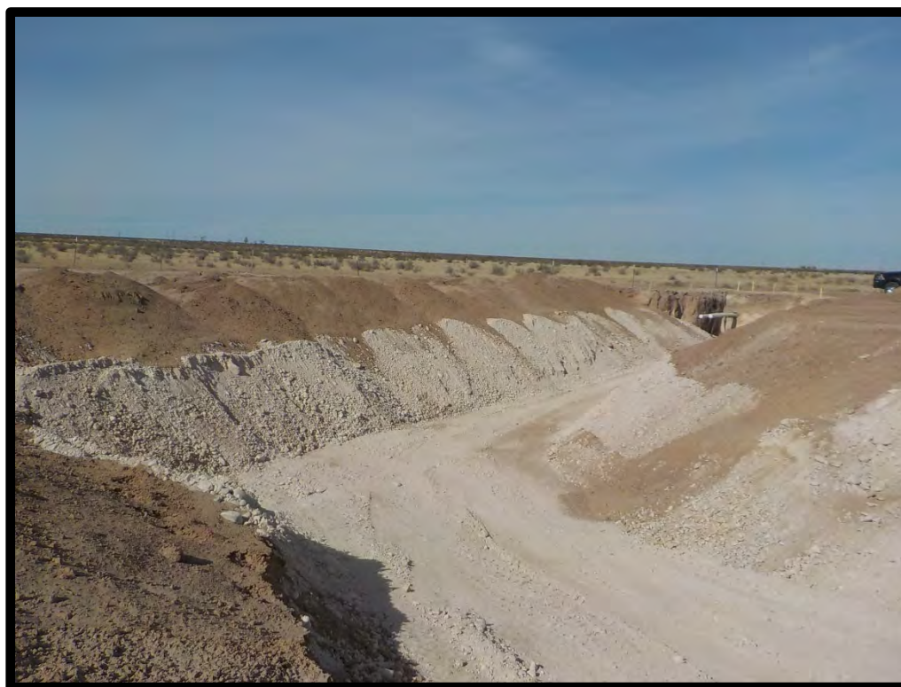
PHOTOGRAPH NO.16 – A view of Western Impact/Excavation Area during the backfill process. The view is towards the northwest (Approximate GPS coordinates 32.682437, -104.500304)
