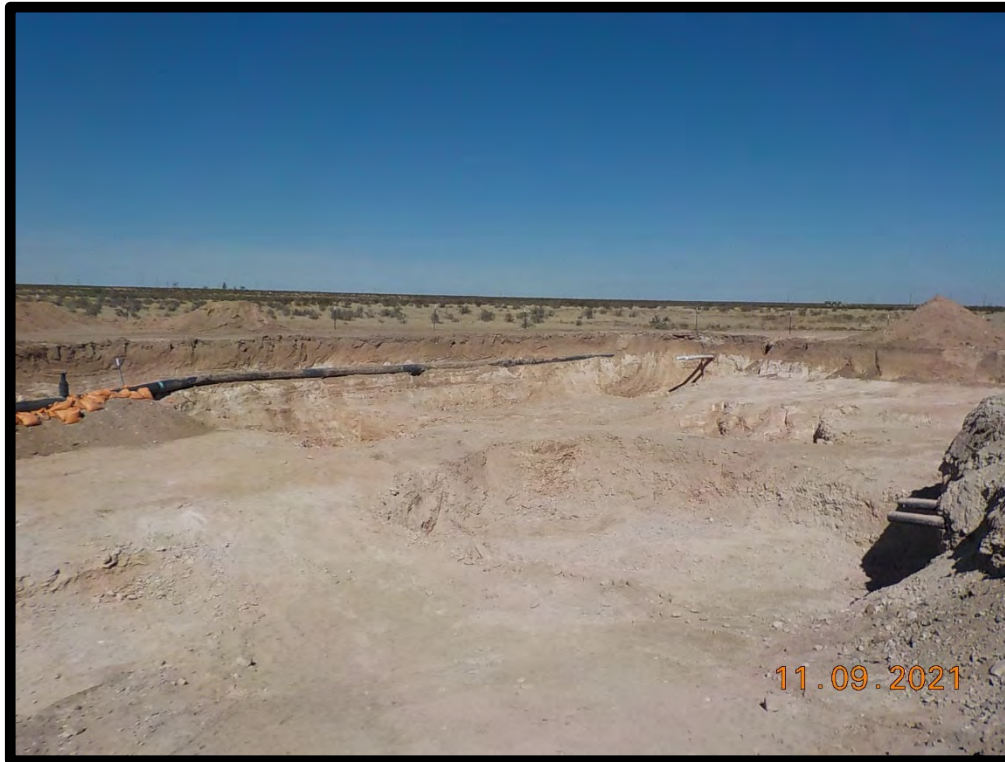
PHOTOGRAPH NO.12 – A general view of the excavated Western Impact/Excavation Area. (Approximate GPS coordinates 32.682534, -104.500053)
