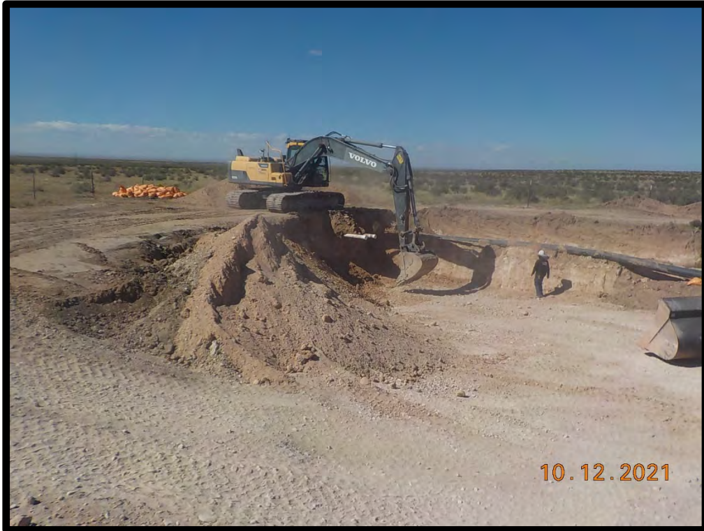
PHOTOGRAPH NO. 9 – A view of the on-going soil removal operations on October 12, 2021. The view is towards the southwest. (Approximate GPS coordinates 32.682527, -104.500060)
