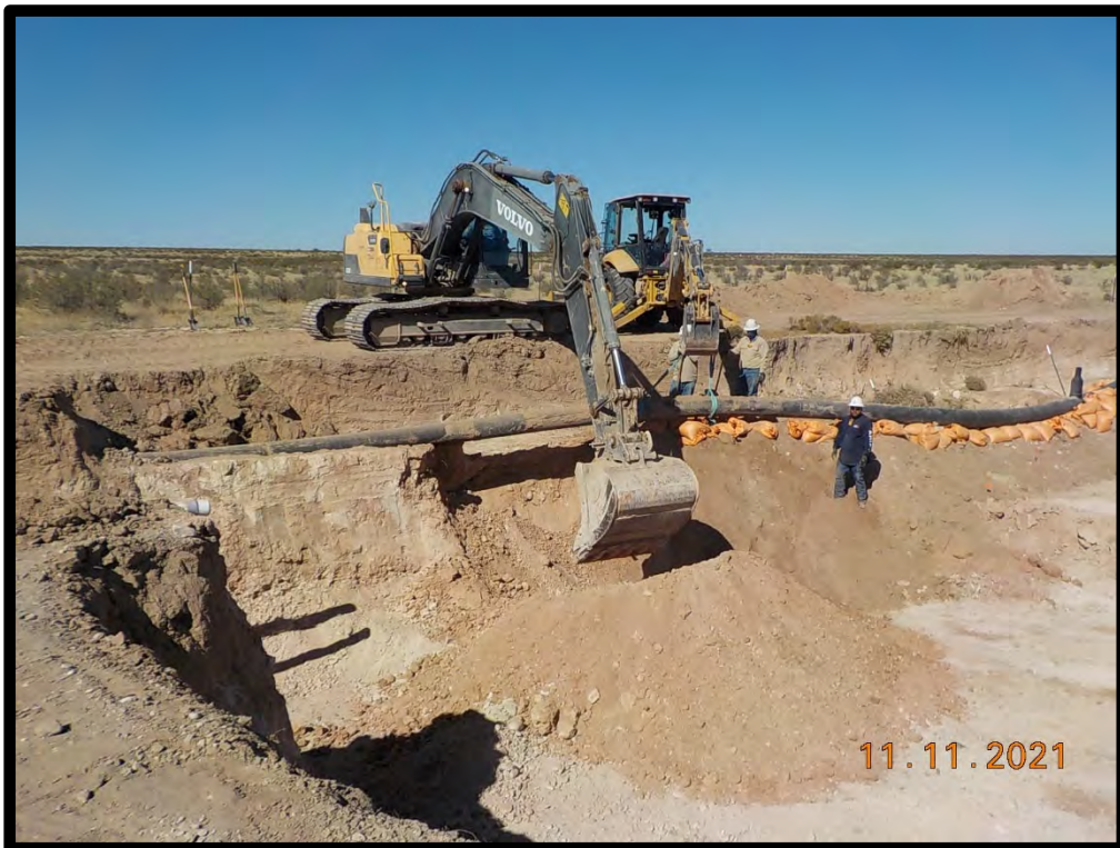
PHOTOGRAPH NO. 10 – A view of soil removal operations along below the high-pressure gas line. The view is towards the west-northwest (Approximate GPS coordinates 32.682464, -104.500218)
