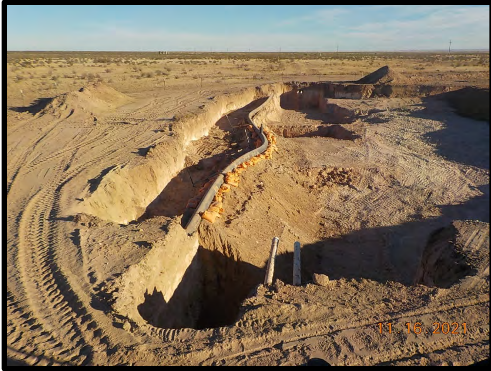
PHOTOGRAPH NO. 13 – A view of Western Impact/Excavation Area during the remedial process. The view is towards the north. (Approximate GPS coordinates 32.682437, -104.500304)
