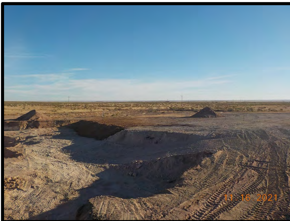
PHOTOGRAPH NO. 15 – A view of Eastern Impact/Excavation Area during the backfill process. The view is towards the east-northeast. (Approximate GPS coordinates 32.682437, -104.500304)
