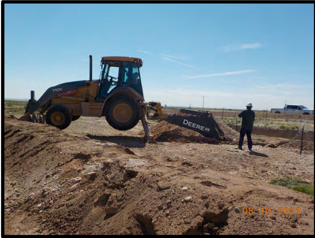
PHOTOGRAPH NO. 7 – A view collected during the August 10, 2021 assessment activities. The view is towards the southeast. (Approximate GPS coordinates 32.682732, -104.499857)
