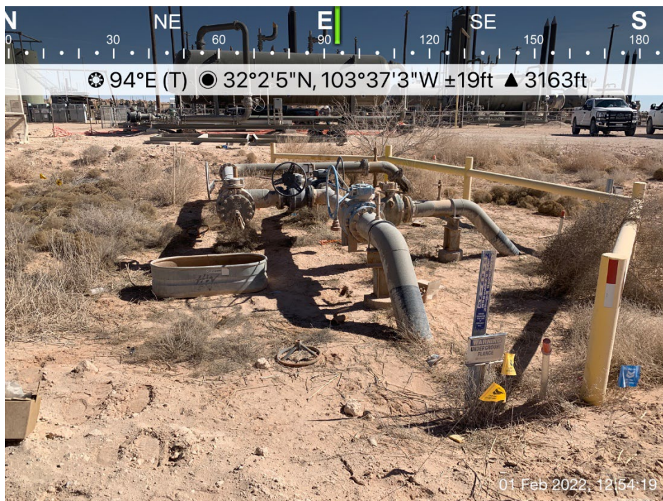
Manifold Release Impacted Area, Viewing East
