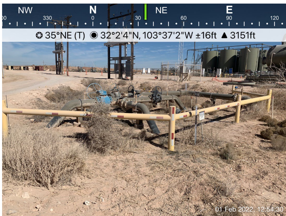
Manifold Release Impacted Area, Viewing Northeast
