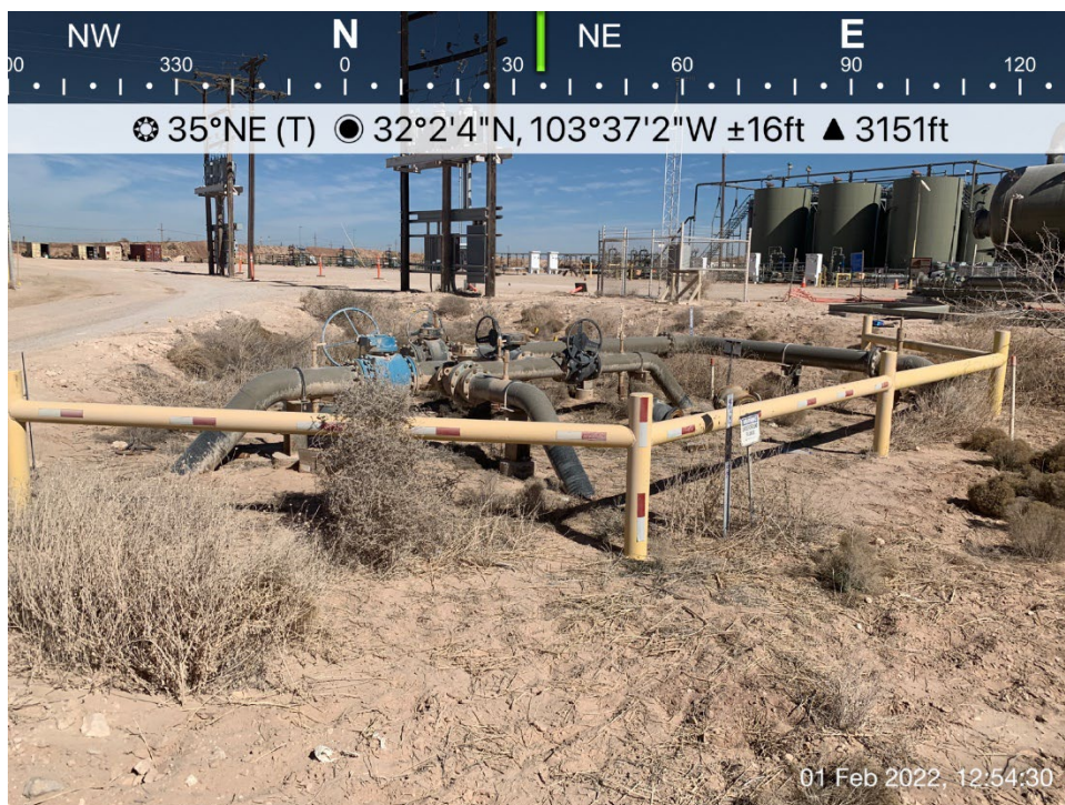
Manifold Release Impacted Area, Viewing Northeast
