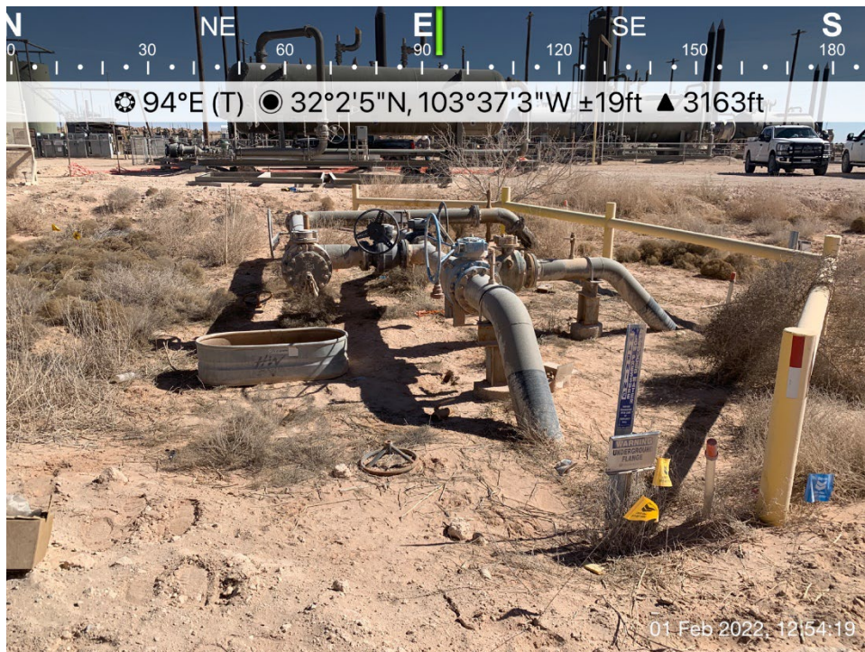
Manifold Release Impacted Area, Viewing East
