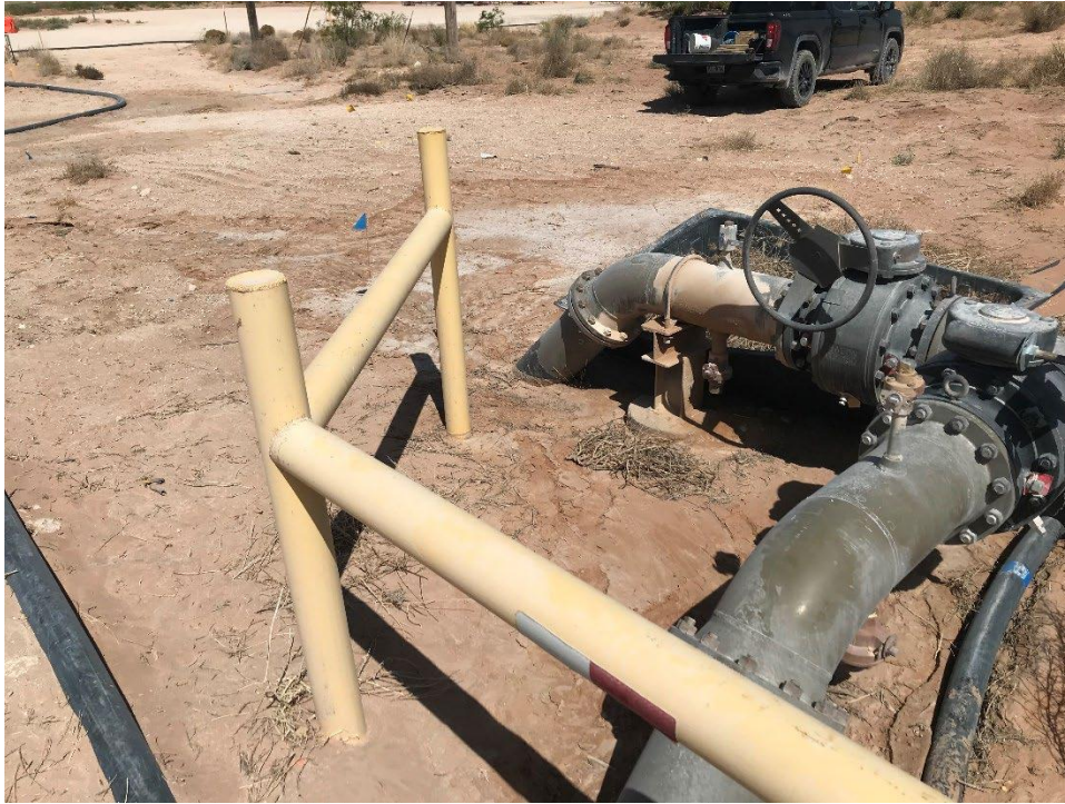
Impacted area (nAPP2211732512) viewing northwest, April 18, 2022
