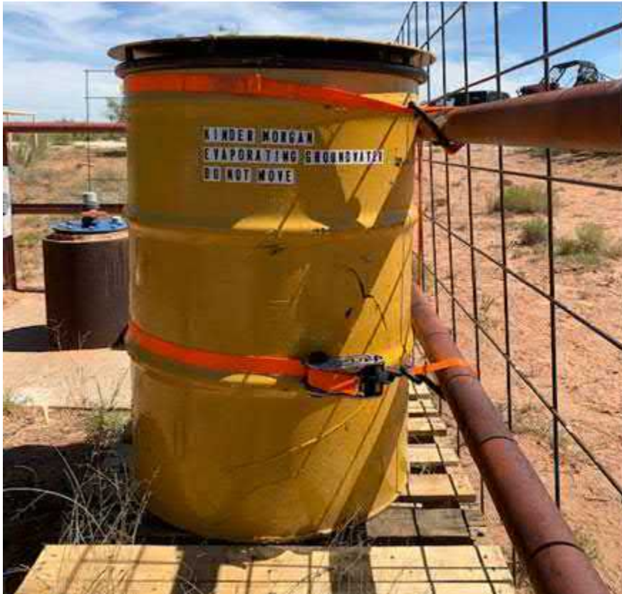
Jal #4 Gas Plant, Jal, New Mexico - Field-Deployed Drum with Ventilated Barrel Cover – Successfully evaporates groundwater monitoring IDW purgewater “24-7”
