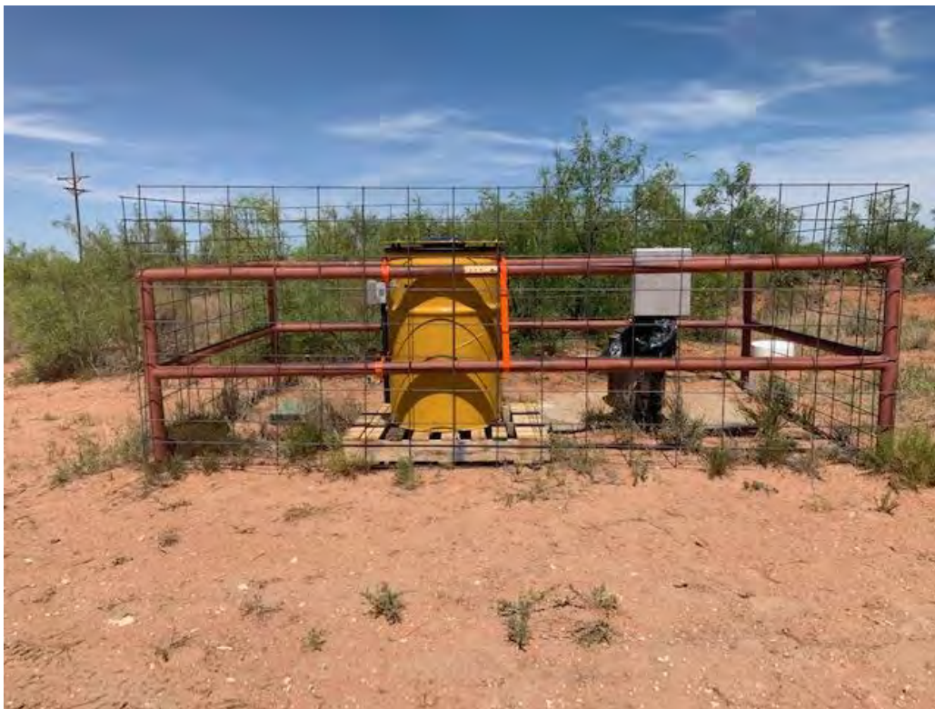
Jal #4 Gas Plant, Jal, New Mexico - Field-Deployed Drum with Ventilated Barrel Cover (Well RW-2 Enclosure)
