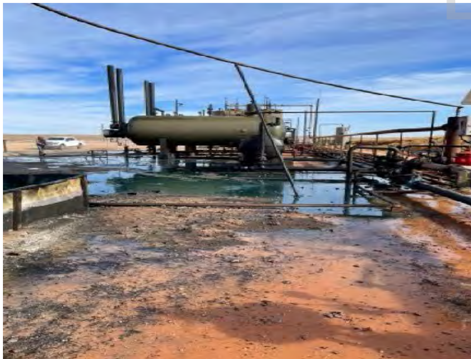
Photo 5: View of free liquids within containment area facing east showing central part of release area. Note containment for the day tank on the left.
