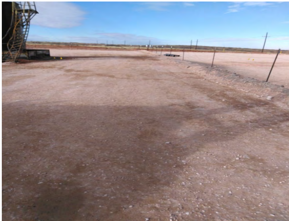
Photo 12: View of release area staining facing west
