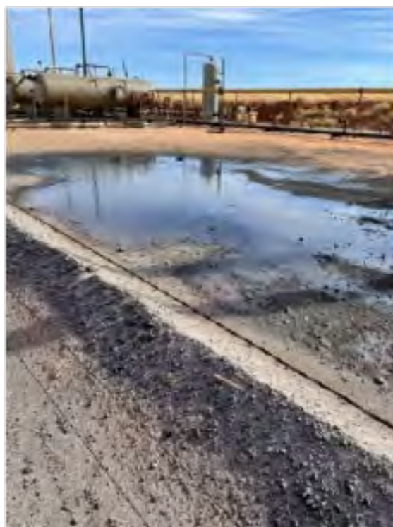
Photo 4: View taken from the central part of the release area facing east-southeast showing free liquids within containment along the northern margin of the release area.
