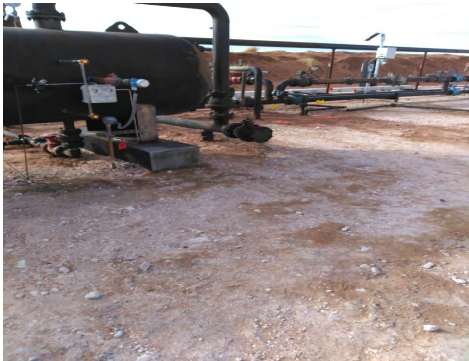
Photo 13: View of release area staining around vessels and piping facing south-southwest
