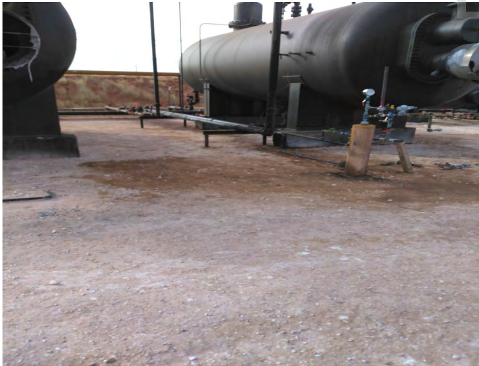
Photo 15: View of release area staining around vessels facing south-southwest.
