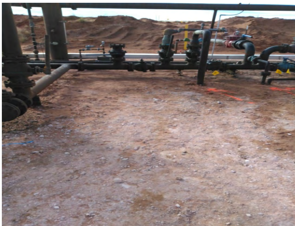
Photo 14: View of release area staining around piping facing south
