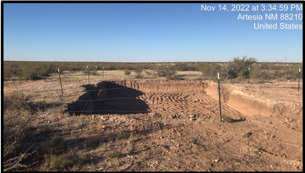
PHOTOGRAPH NO. 2 – A view of the northern excavation/remediation area at the Site upon completion of the soil removal operations. The view is towards the north.
