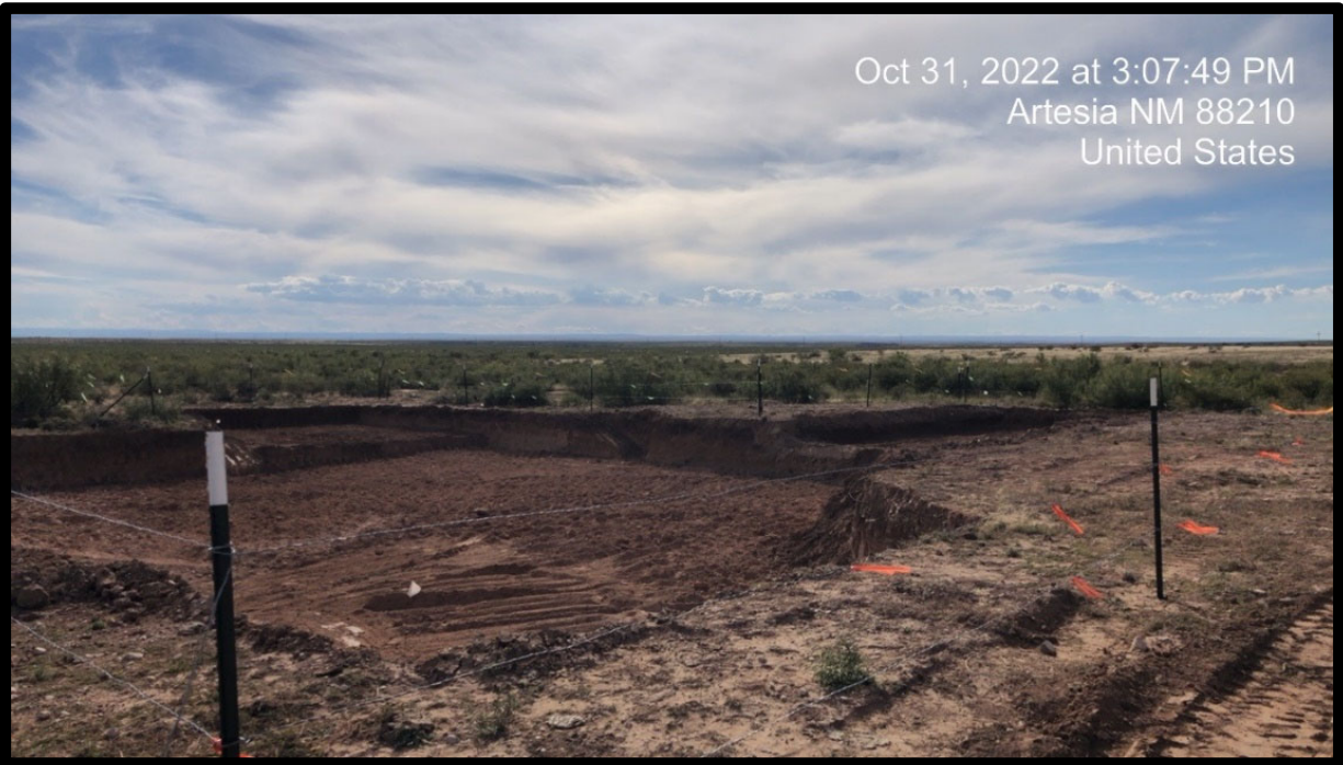
PHOTOGRAPH NO. 1 – A view of the southern excavation/remediation area at the Site upon completion of the soil removal operations. The view is towards the southwest.
