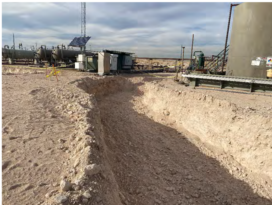
View of Ex-5 observed at the site on December 1, 2021. View is towards the northwest.
