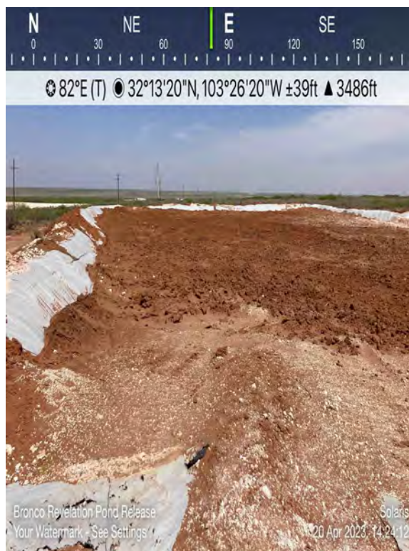
View of Treatment Cell– View East
