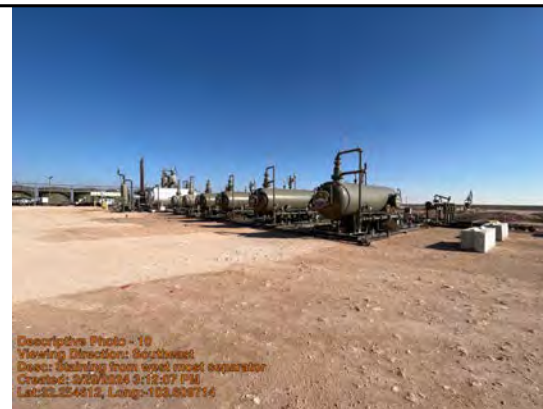
Staining from west most separator
