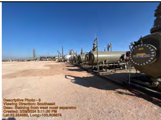
Staining from west most separator
