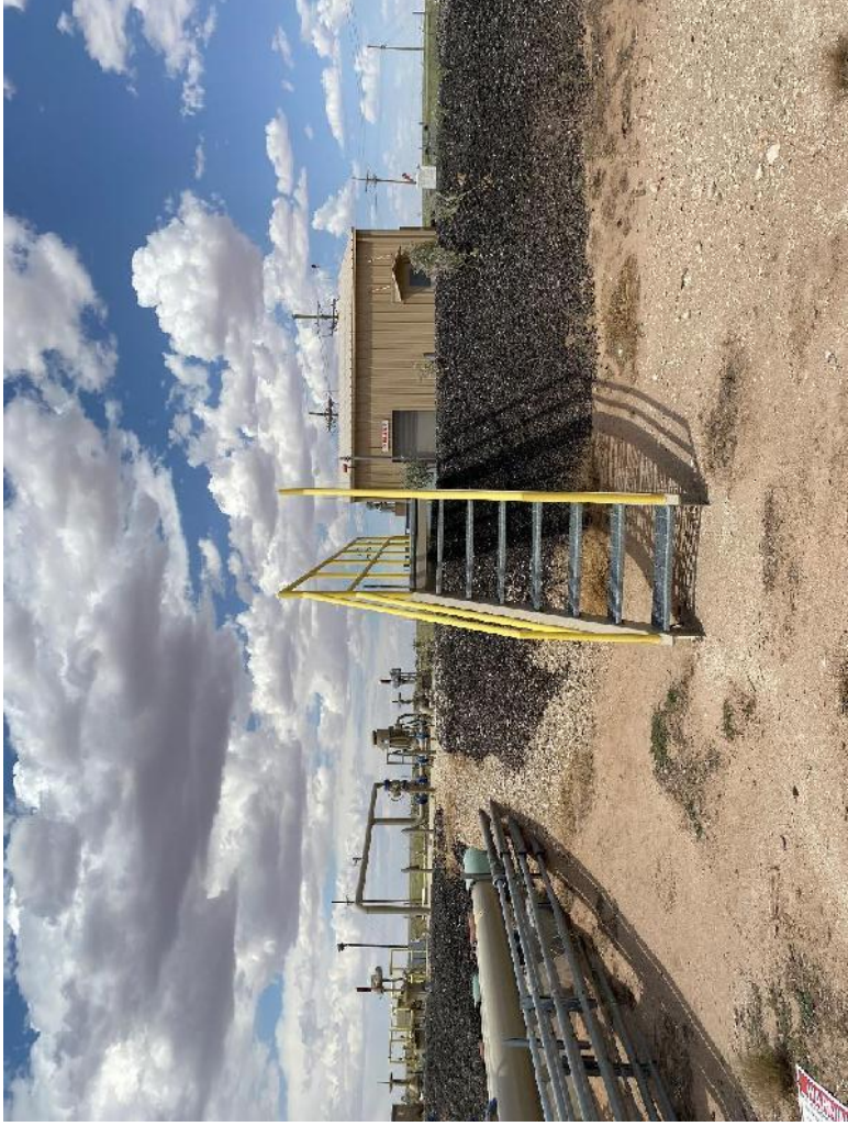
Photograph location 17. August 22, 2024. Central portion of the facility, inside northern berm of former Tank 970 facing north. View of aboveground piping and stairs that pass through and over the berm, respectively.
