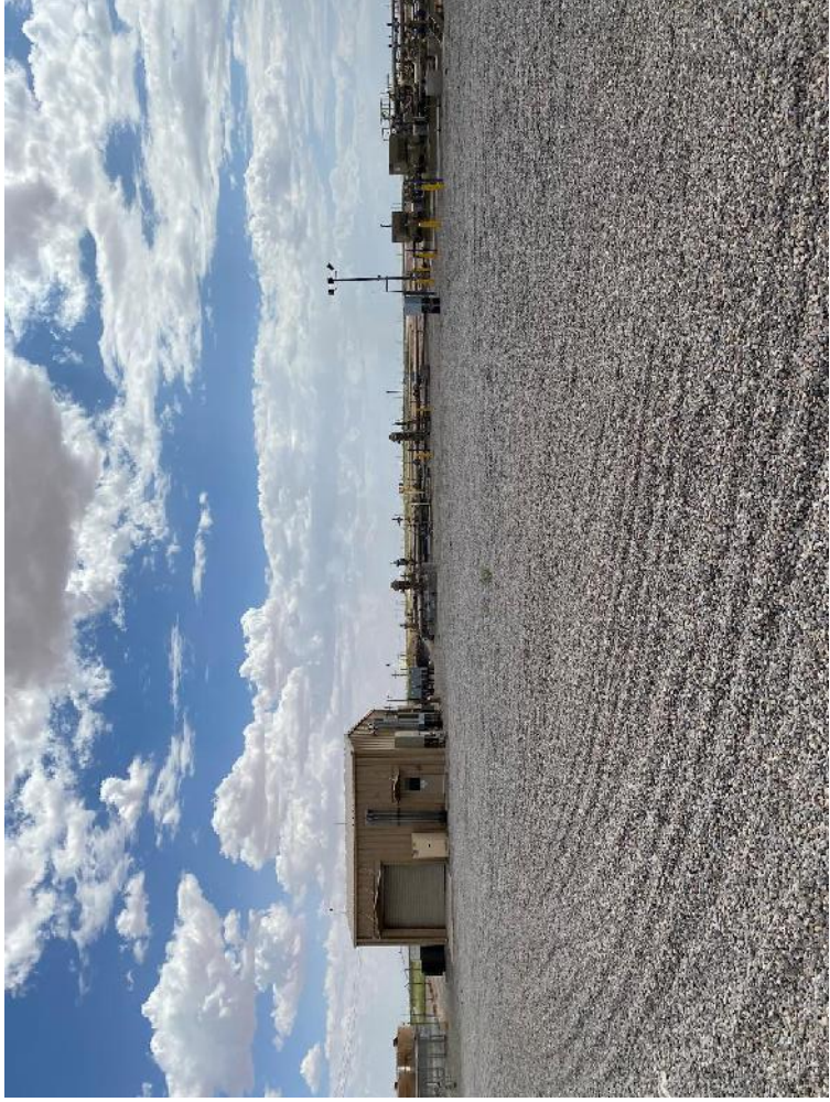
Photograph location 3. August 22, 2024. North portion of facility, facing south overlooking SB-North location. View of aboveground pipelines, structures and equipment between SB-North and release area.
