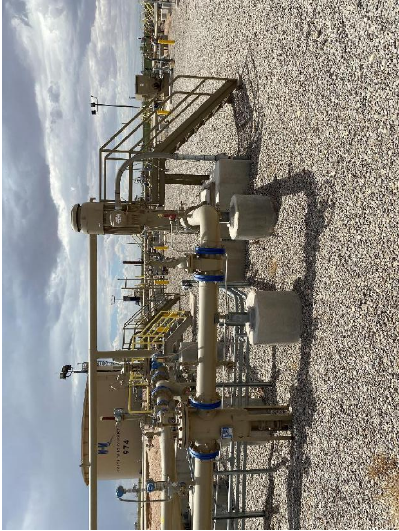
Photograph location 9. August 22, 2024. Central portion of the site, just north of the berm and aboveground piping located north of the release/excavation area facing west. View of aboveground pipelines and supports.
