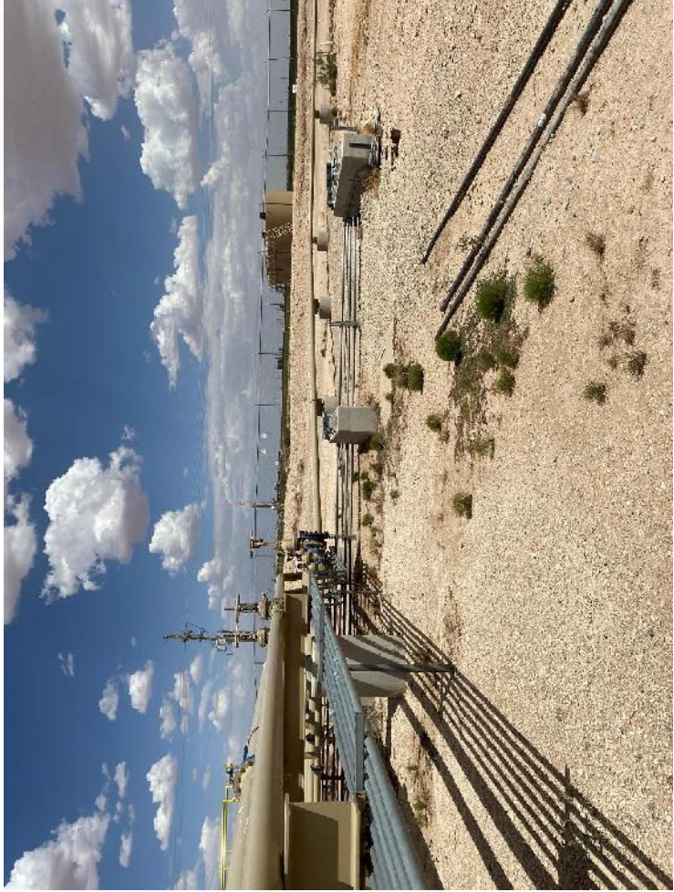
Photograph location 20. August 22, 2024. Central portion of the facility, inside northern berm of former Tank 970 facing east. View of HA-North location and adjacent aboveground pipelines and concrete supports.
