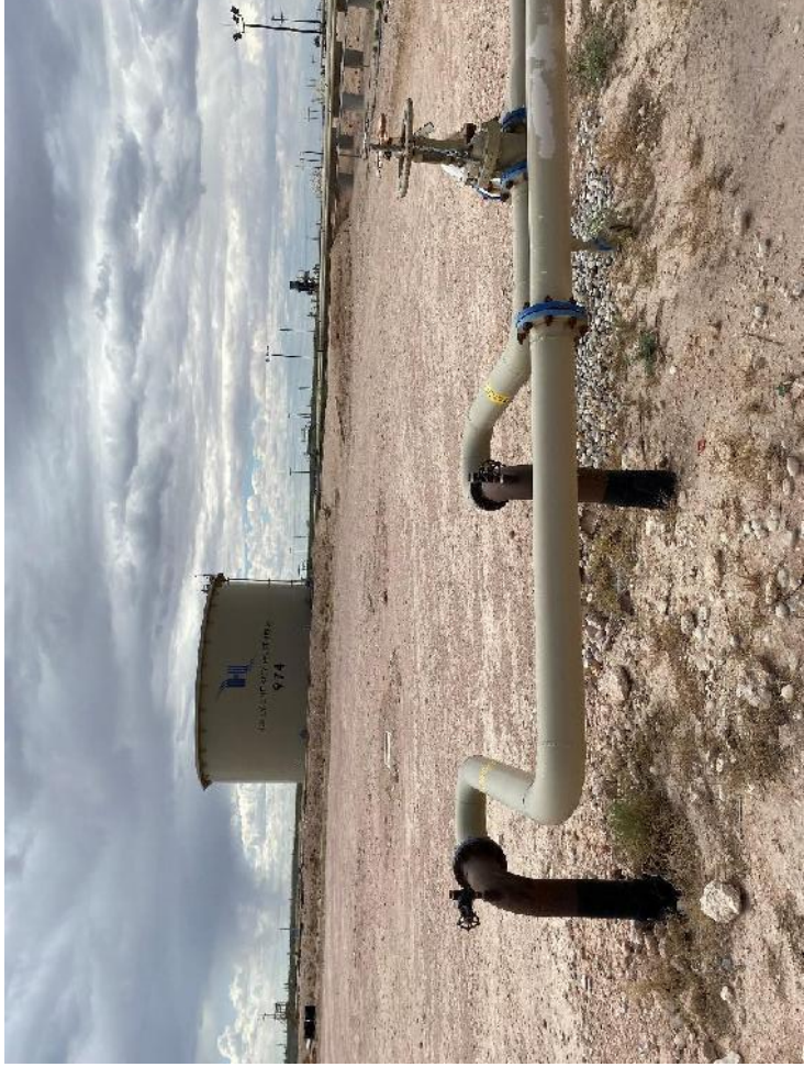
Photograph location 36. August 22, 2024. Facing west. View of aboveground pipelines located near the berm surrounding former Tank 970.
