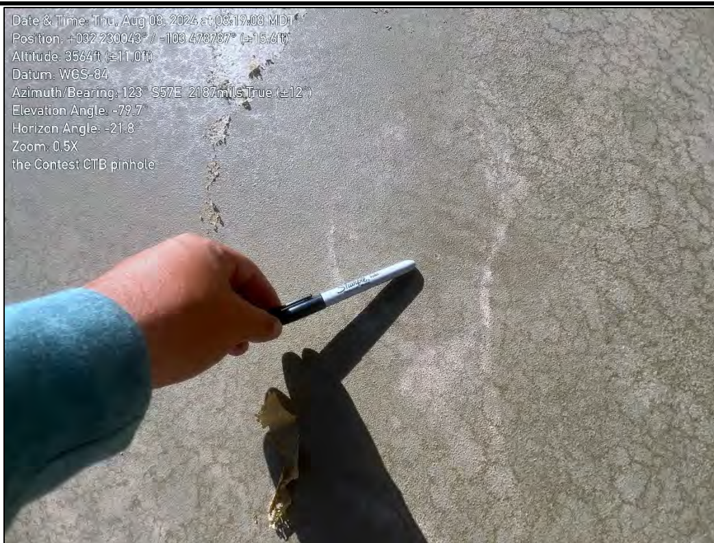
PHOTO 6: Southeast view of potential pinhole during liner inspection activities. 8/08/2024
