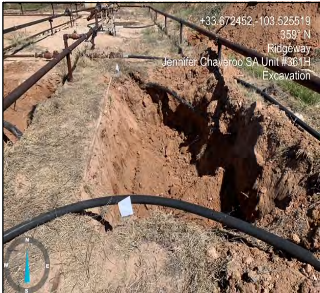
Photograph showing the depth and the progress of the excavation facing North.
