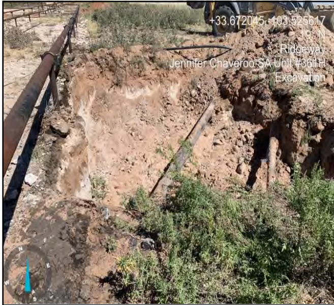
Photograph showing the depth and the progress of the excavation facing North.
