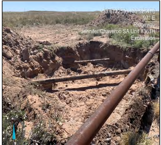
Photograph showing the depth and the progress of the excavation facing East.
