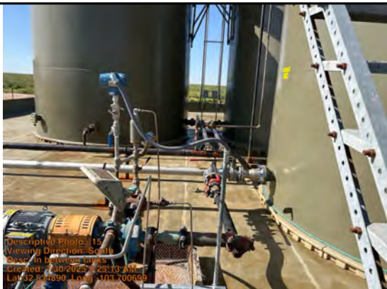
In between tanks
