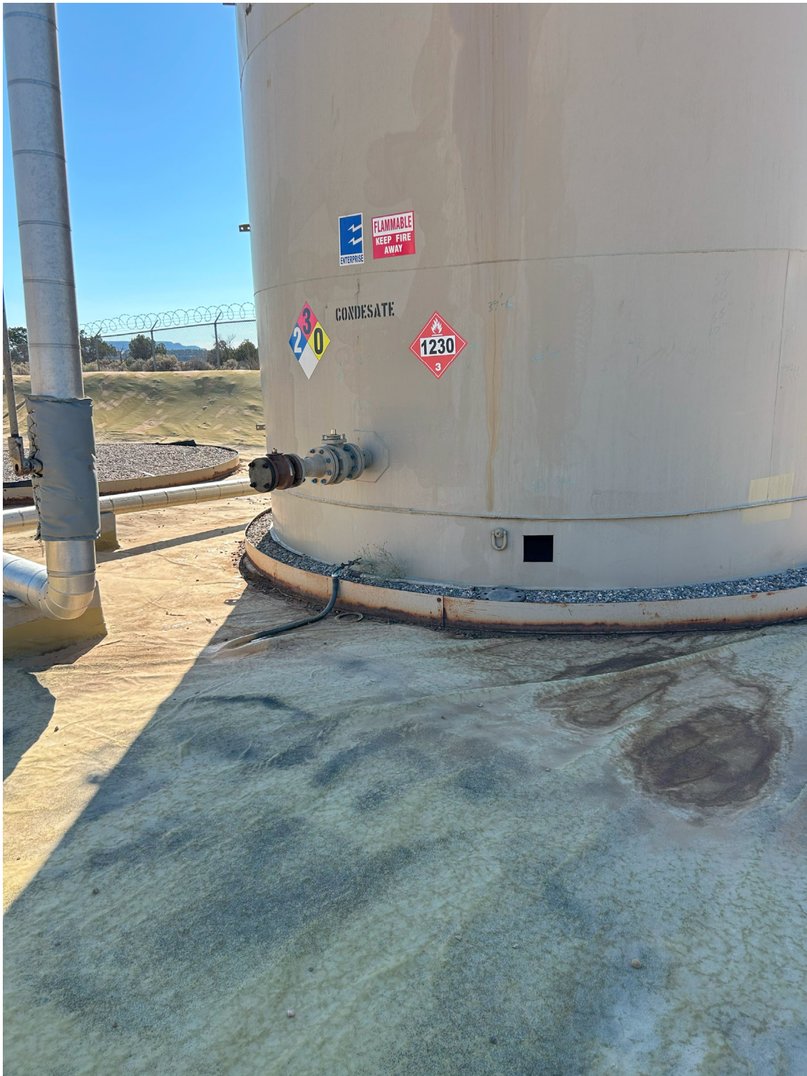
Photo 1: View of the 500 BBL tank inside the secondary containment system.
