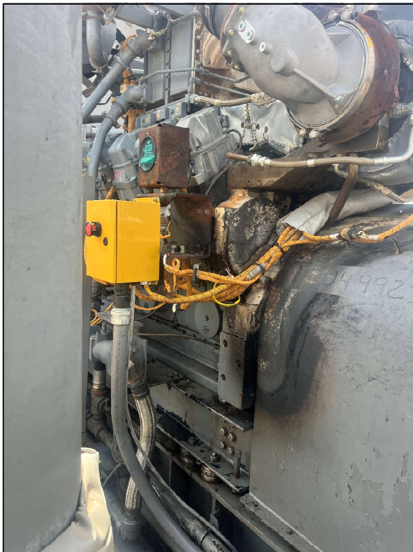
Photo of unit 804992 after the replacement of equipment following the event
