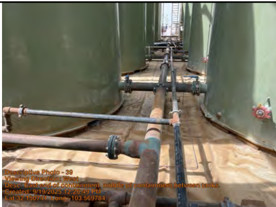
East end of containment, middle of containment between tanks.
