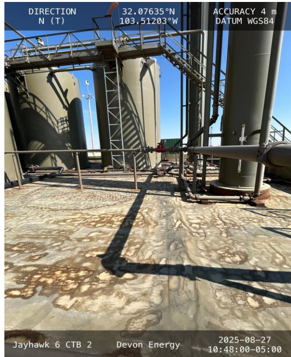
Photo 8 View of eastern portion of secondary containment facing north.
