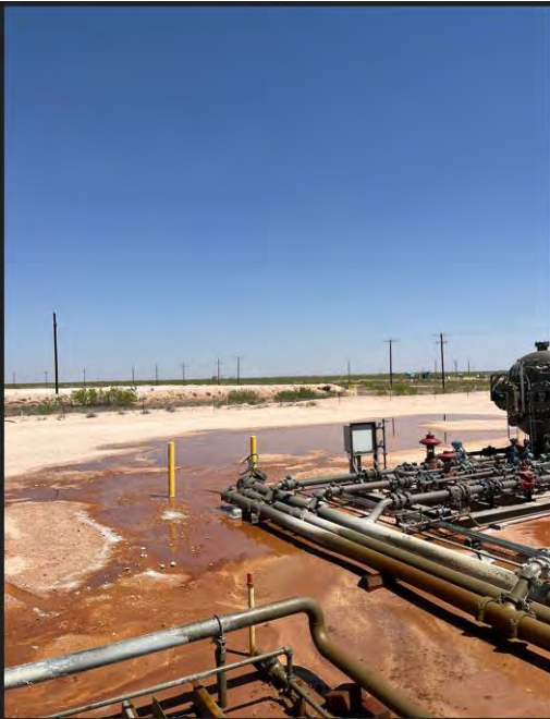
Photograph 1 Date: 4/16/2025 Description: Spill area (nAPP2510725008) View: Northeast
